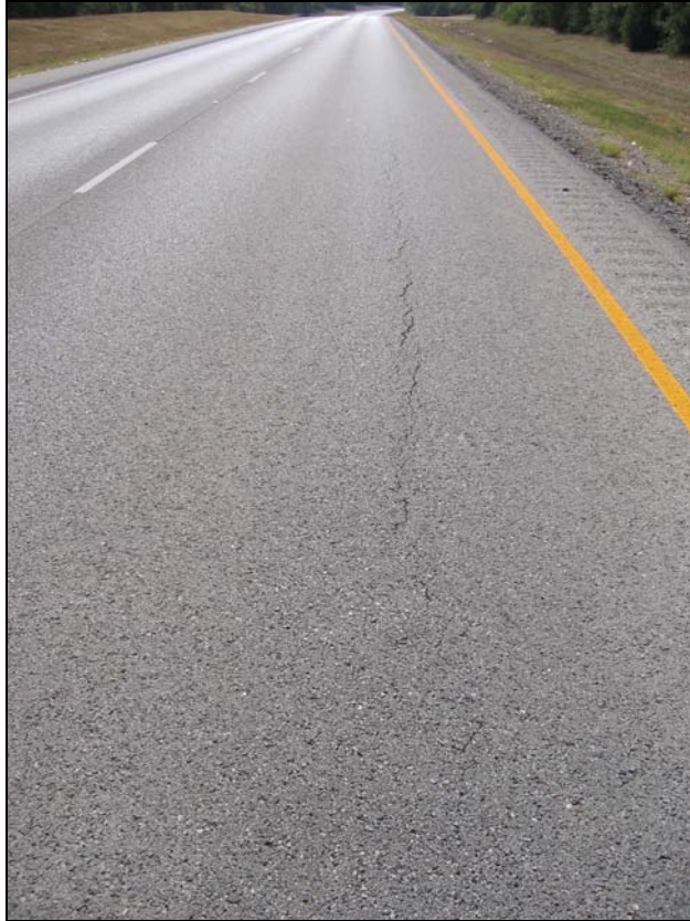
Figure 1.4. Longitudinal Crack in SH 47 NB from STA 1161.33 to 1160.95.
