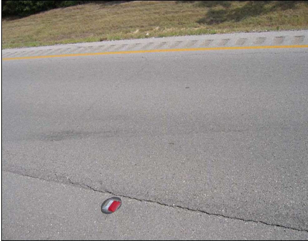
Figure 1.8. Cracking in SH 47 SB from STA 2144.94 to 2145.66
