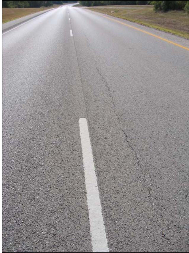
Figure 1.3. Longitudinal Crack in SH 47 NB from STA 1163.70 to 1163.10.
