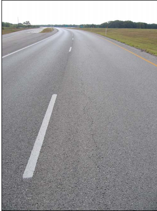
Figure 1.2. Second Longitudinal Crack in SH 47 NB.
