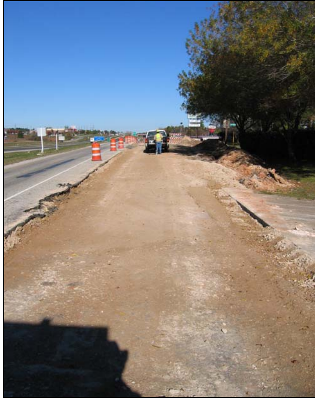
Figure 3.3. Looking North from the Start of the NB IH 45 Frontage Road Project.
