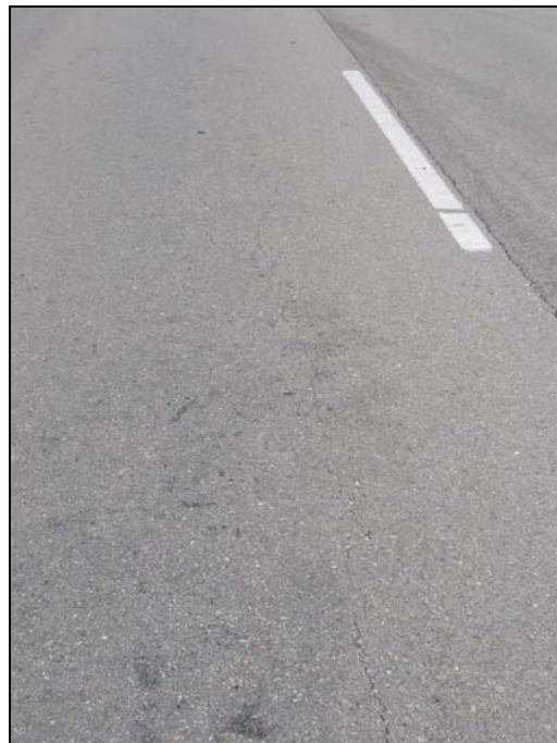
Figure 1.9. Cracking in SH 47 OL from STA 2145.23 to 2145.43 (Joint crack from 2144.80 to 2145.70 also visible).
