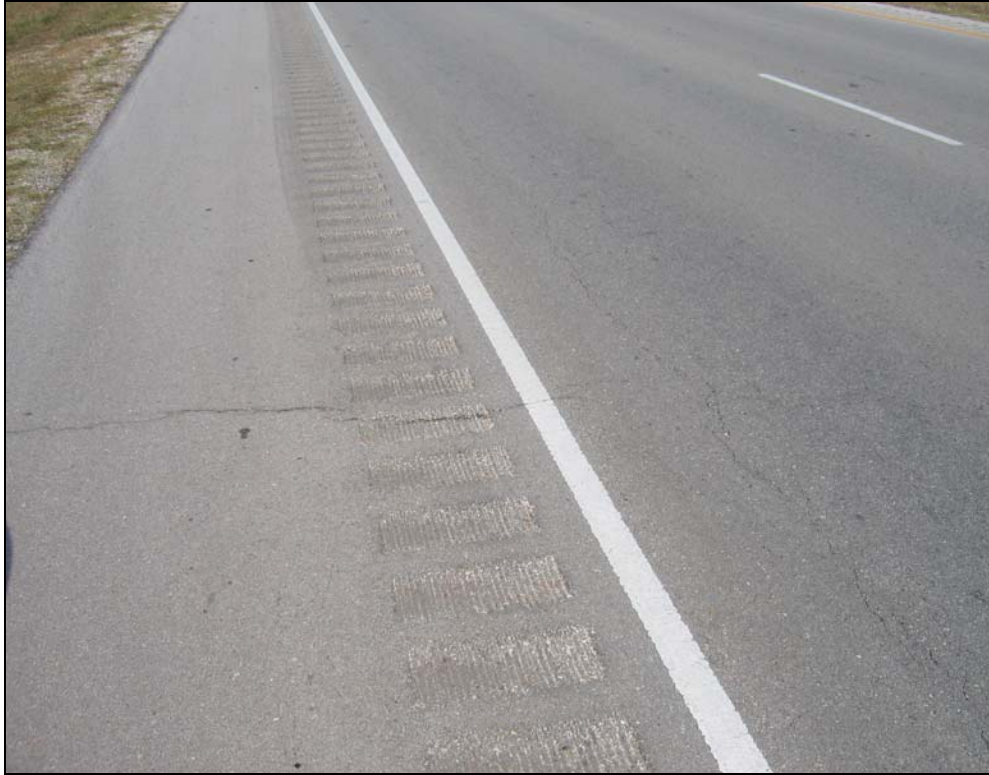
Figure 1.14. Cracking in SH 47 SB from STA 2154.49 to 2154.89.
