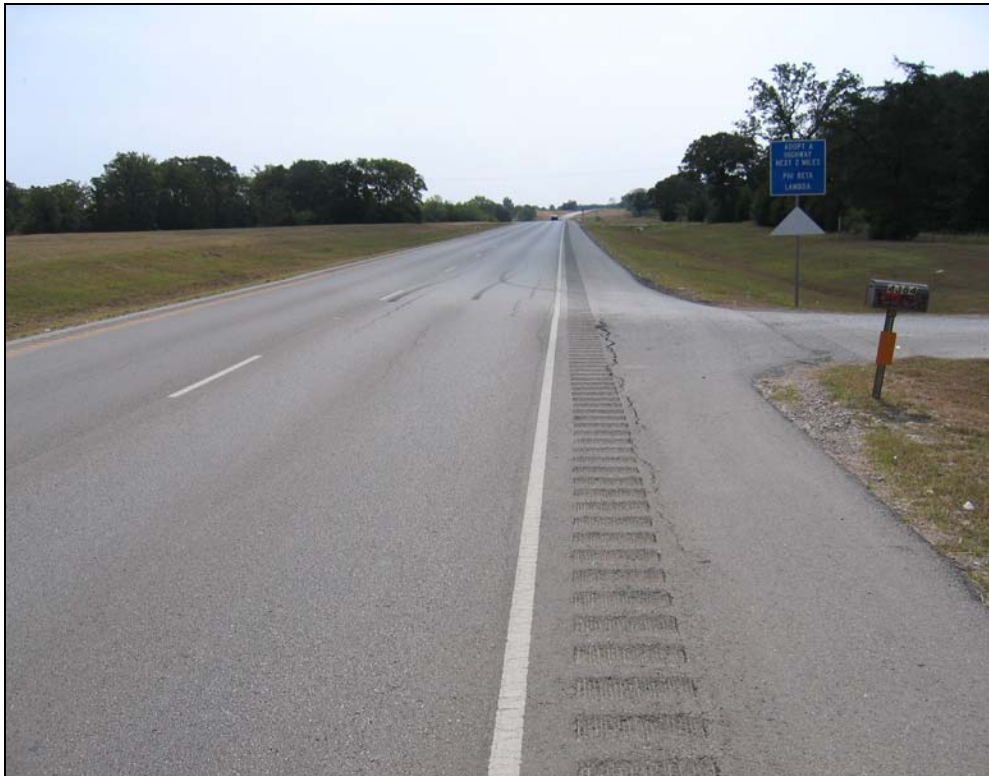
Figure 1.15. Cracking in SH 47 SB from STA 2155.94 to 2156.92.
