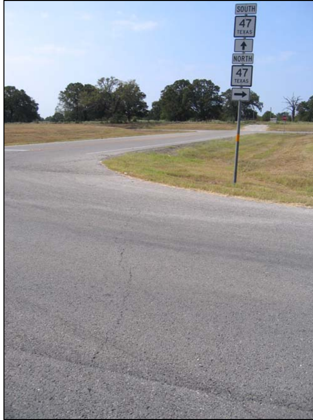
Figure 1.5. Transverse Crack at STA 1124.84 in SH 47 NB.
