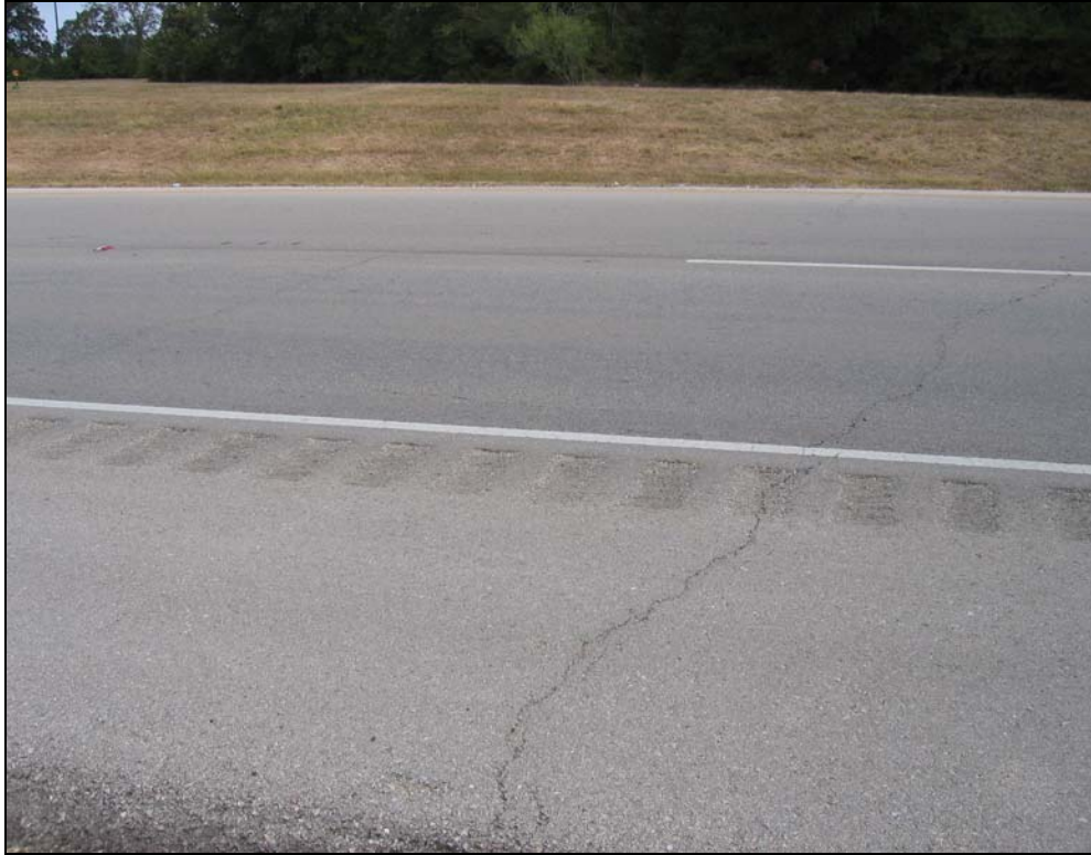
Figure 1.16. Block Cracking in SH 47 SB from STA 2161.88 to 2162.99.
