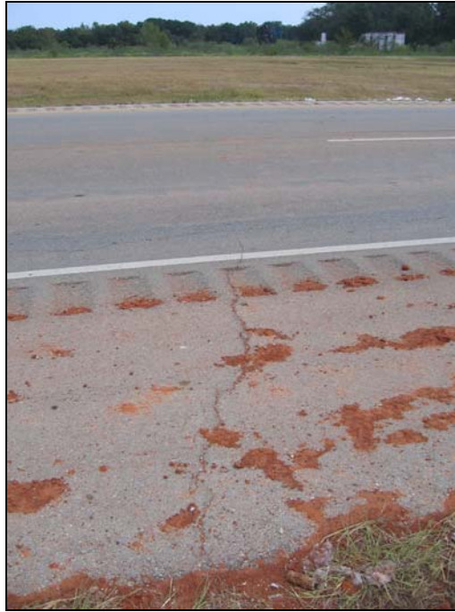
Figure 1.18. Cracking in SH 47 SB from STA 2289.69 to 2290.11.
