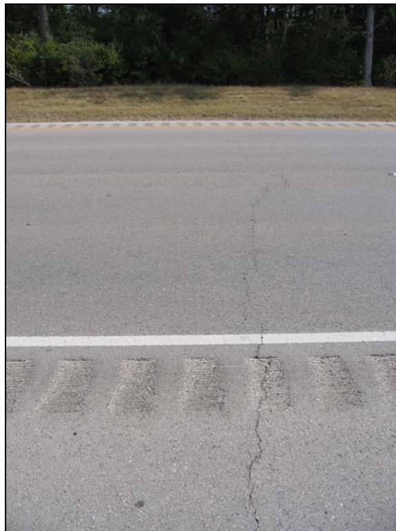
Figure 1.7. Transverse Crack on SH 47 SB at STA 2143.50.
