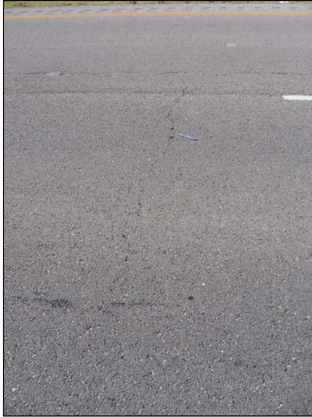
Figure 1.1. First Longitudinal and Transverse Crack on SH 47 NB.
