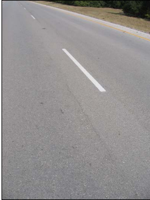
Figure 1.12. Longitudinal Cracking in SH 47 SB OL from STA 2147.72 to 2147.86.
