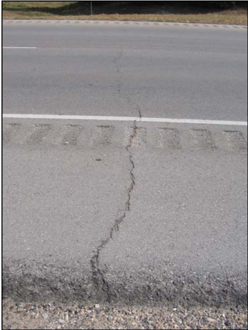
Figure 1.13. Transverse Cracking in SH 47 SB at STA 2153.87.
