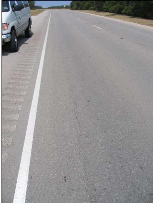
Figure 1.10. Longitudinal Crack in SH 47 SB OL from STA 2146.68 to 2147.20.
