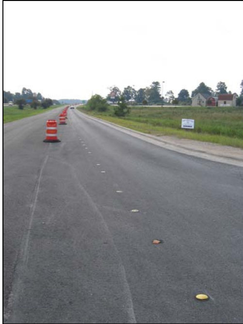
Figure 3.6. Looking South from Veterans Memorial Parkway in Microcracked Section, August 2005.
