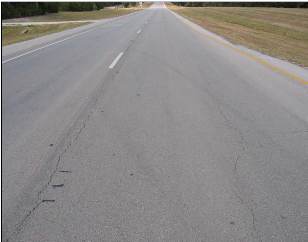
Figure 1.17. Cracking in SH 47 SB OL from STA 2146.06 to 2146.86.
