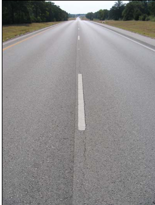
Figure 1.6. Distress on SH 47 SB from STA 2142.52 to 2143.06.
