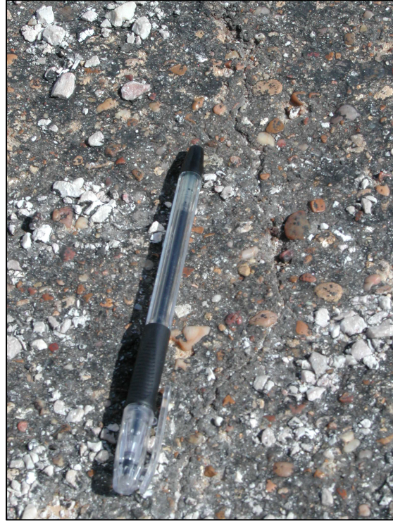
Crack in section microcracked.
