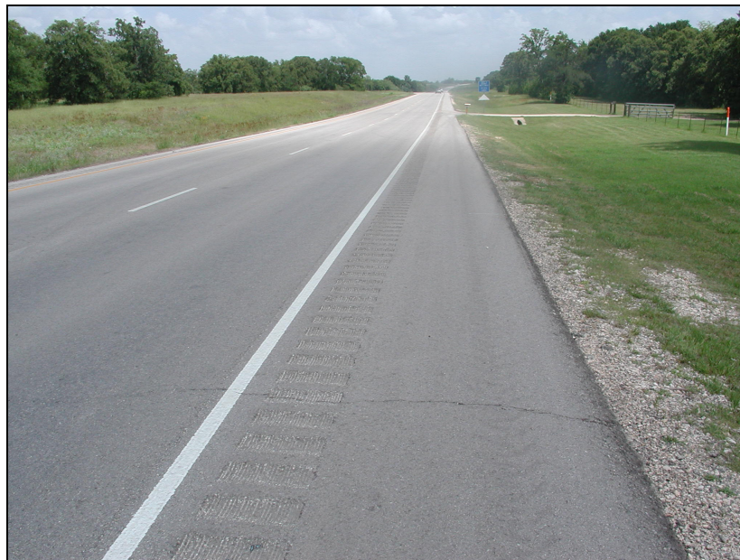
Figure 3.5. Transverse Crack in SB CTB Section on SH 47.
