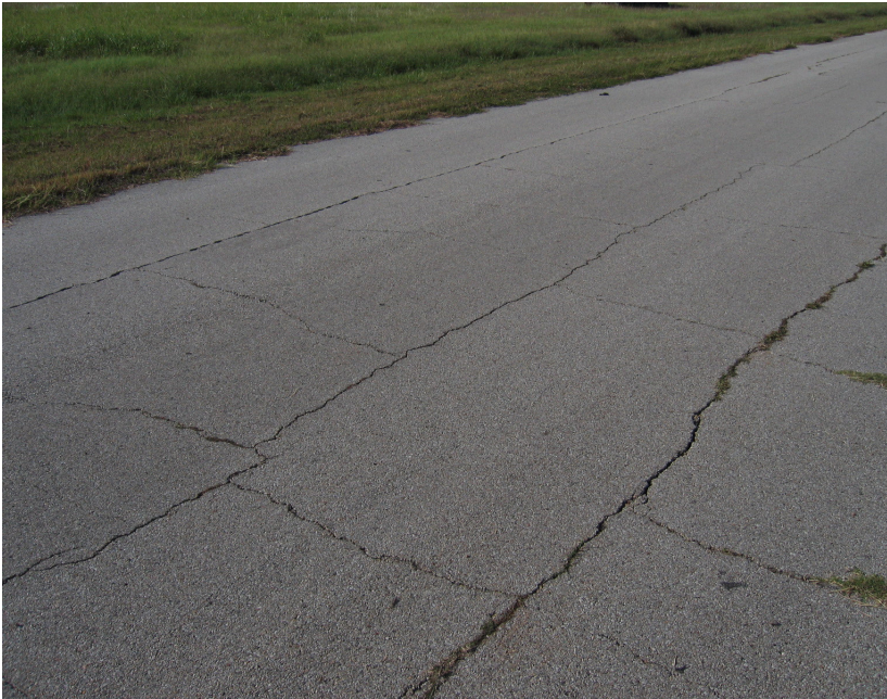
Block cracking typical of CTB.
