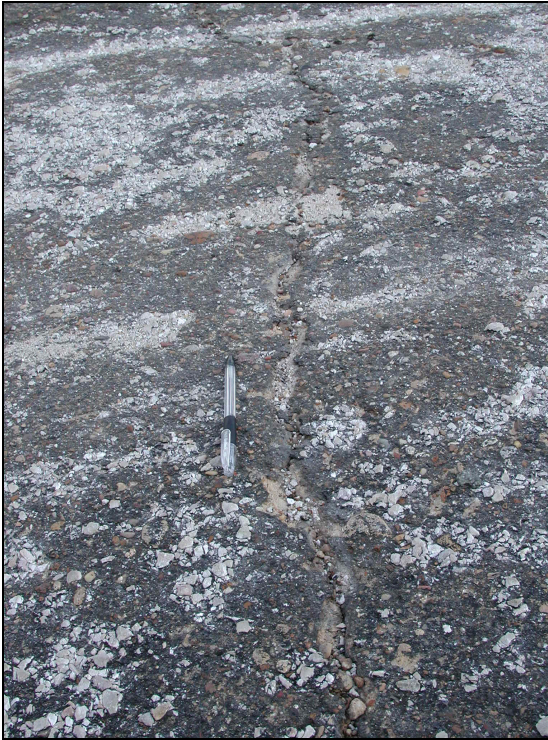
Crack in moist-cured section.
