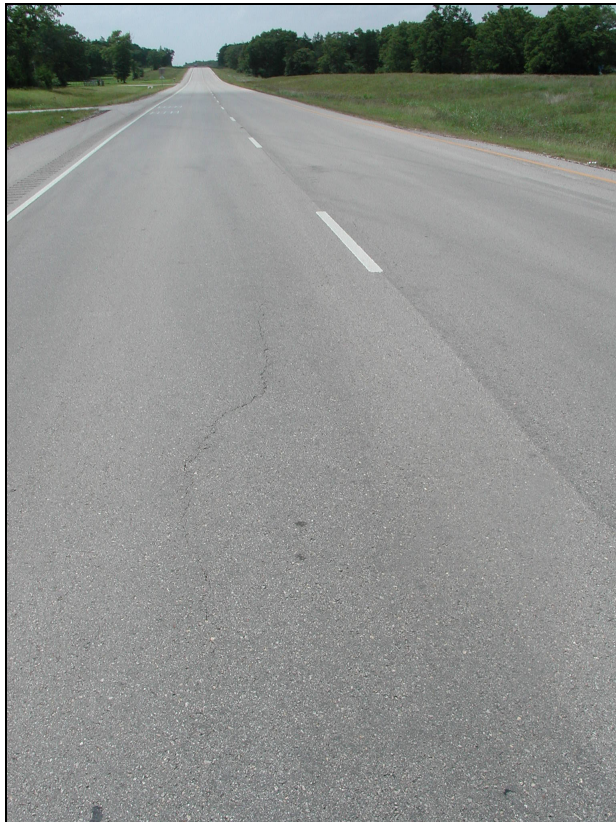
Figure 3.7. Longitudinal Crack on SH 47.
