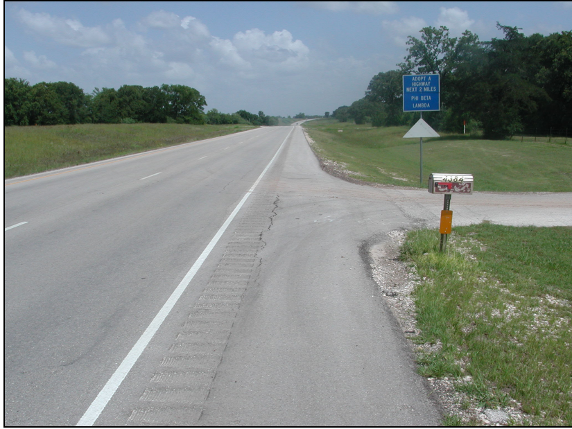
Figure 3.6. Longitudinal Cracking in SB CTB Section on SH 47.
