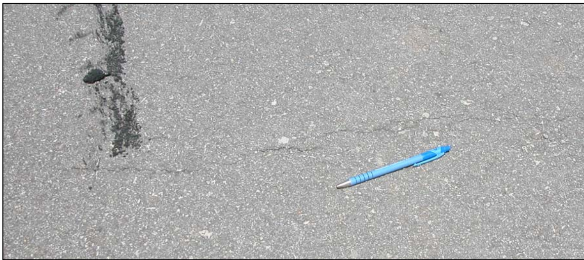
Figure 4.7. Unsealed Crack on SH 16.
