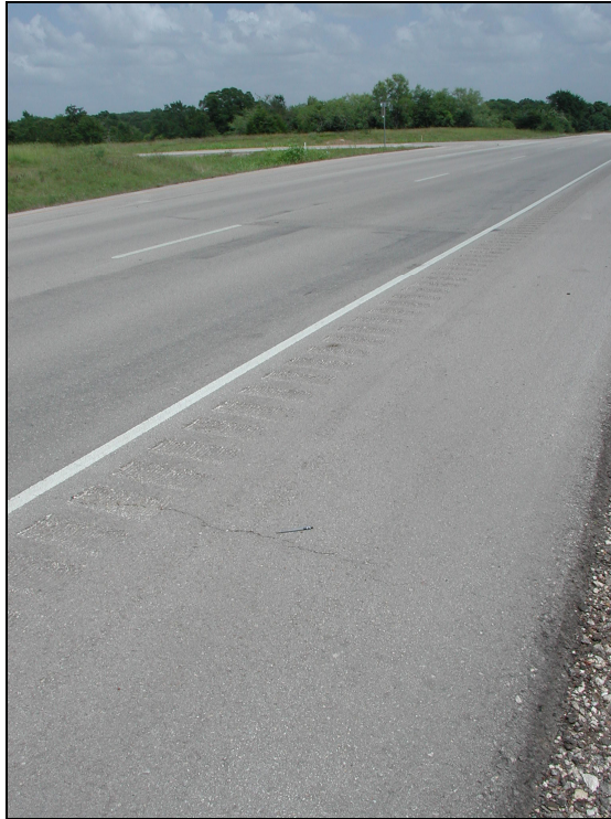
Figure 3.8. Transverse Crack near STA 2164 on SH 47 SB.
