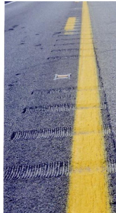
Figure 5. Kentucky's Centerline Rumble Strips.
