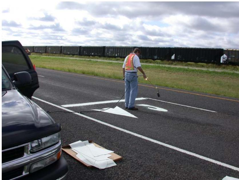
Figure 37. Avery 125 Installation, 2003, Abilene.
