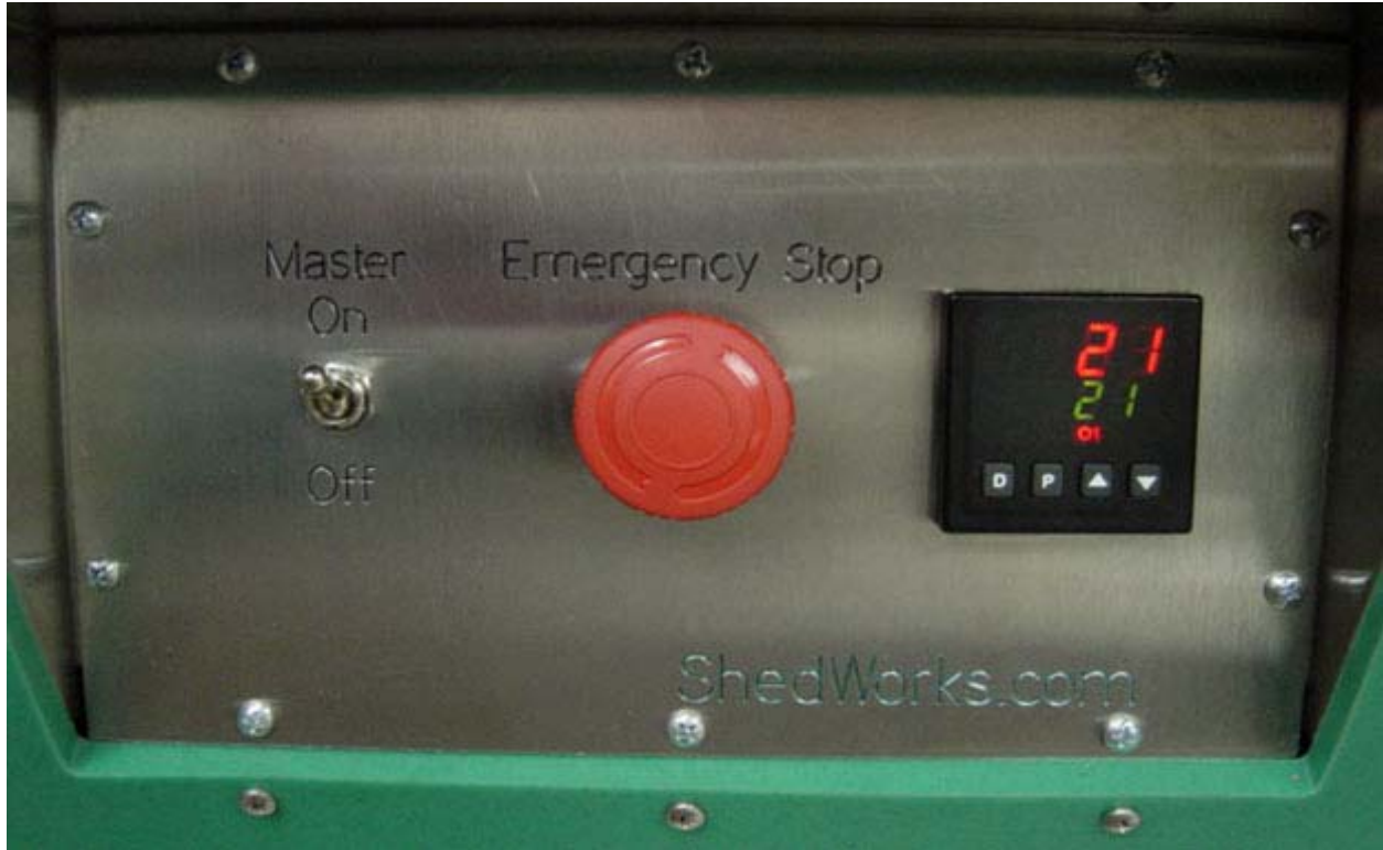
Figure 4. Main Control Panel.
