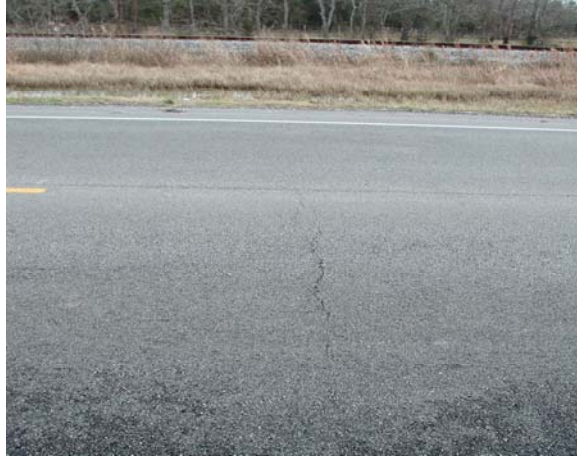
Figure 21. Reflective Cracking in Control Section after One Year of Service.
