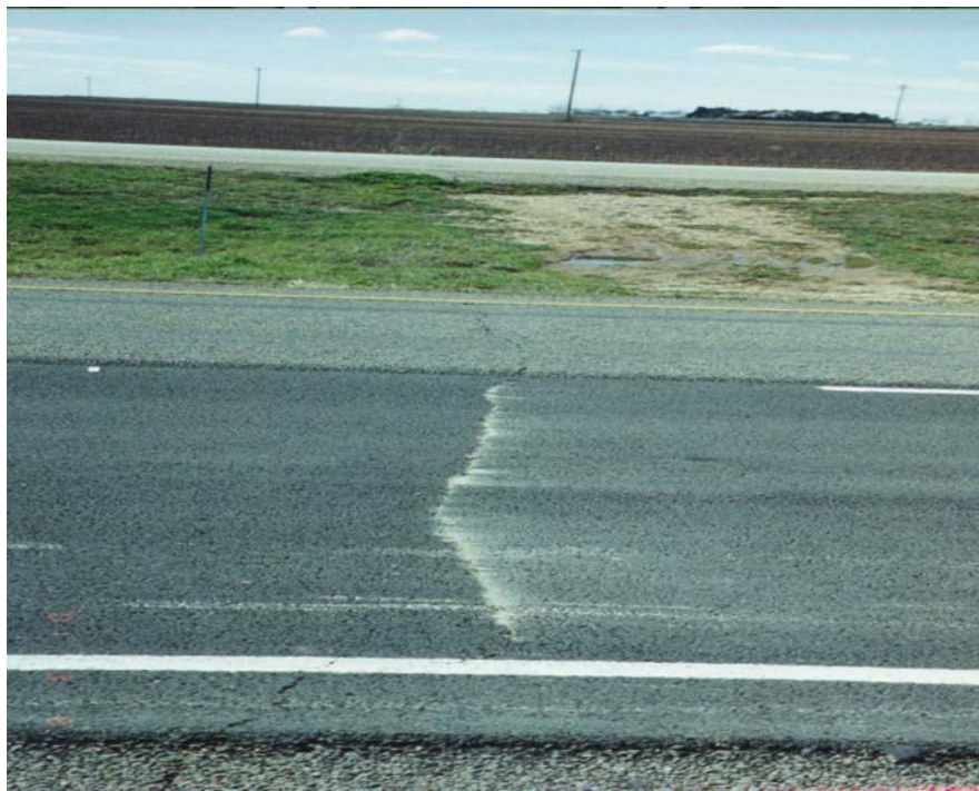
Figure 19. Reflective Cracking on US84 Remixer Section.
