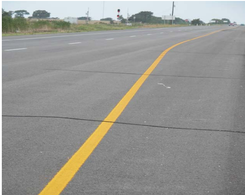
Figure 24. Reflective Cracking on the Left Lane of SH6.
