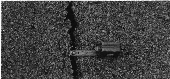
Medium-Severity Longitudinal Cracking
