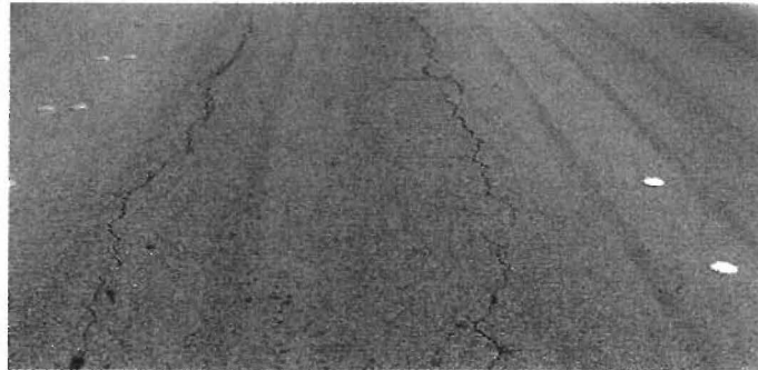
Low-Severity Fatigue Cracking
