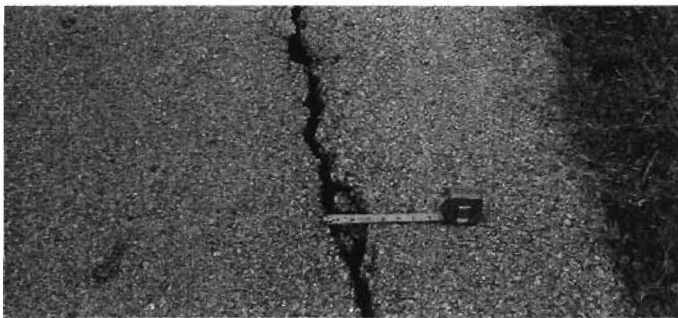
High-Severity Longitudinal Cracking
