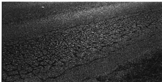
High-Severity Fatigue Cracking
