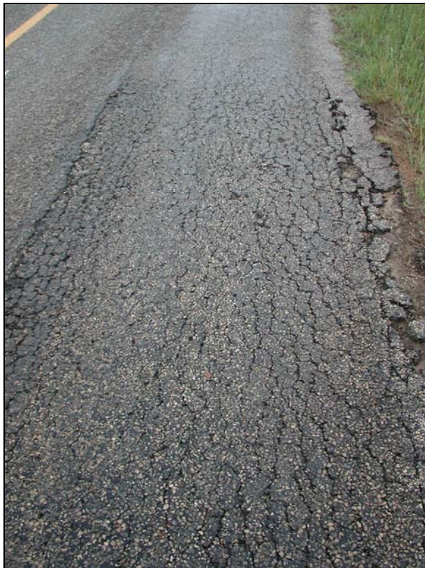
Figure 1.13. FM 3335 Fatigue Cracking.
