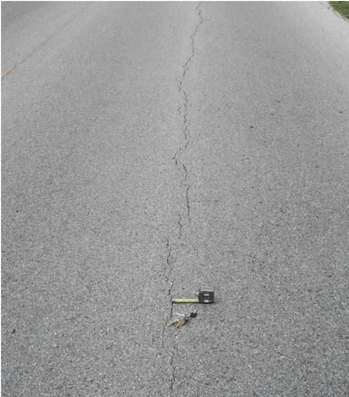
Low Severity Longitudinal Cracking
