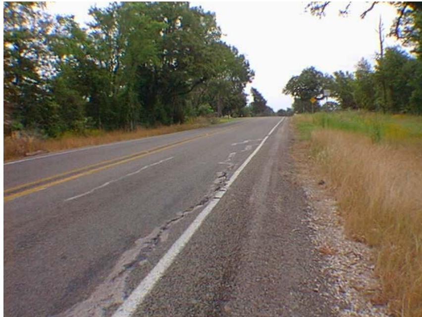
Figure 16. Representative Distresses on OSR.
