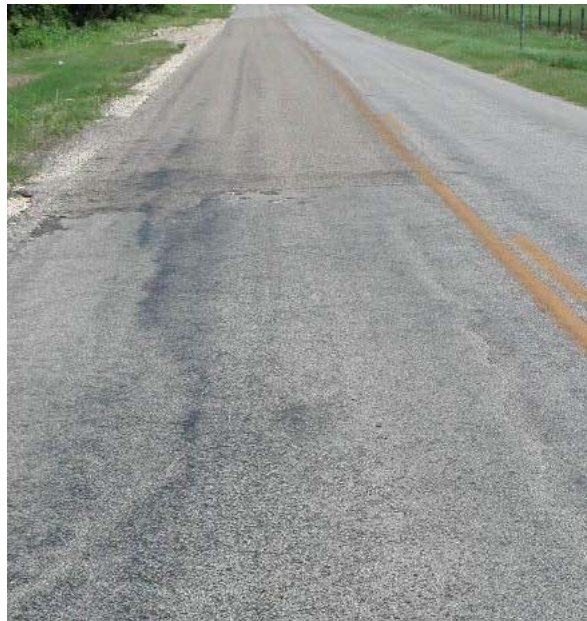
Figure 21. Cracking on FM 20 Section.
