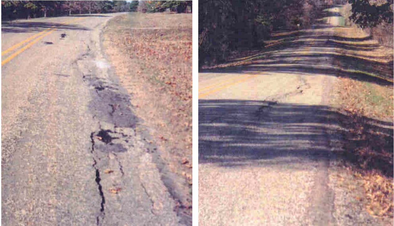
Figure 8. Edge Cracking and Faulting Distresses on FM 2076 before Treatment.
