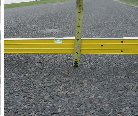
High Severity Rutting
