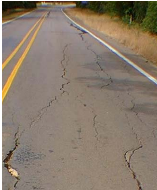
Figure 1. Example of Longitudinal Cracking.
