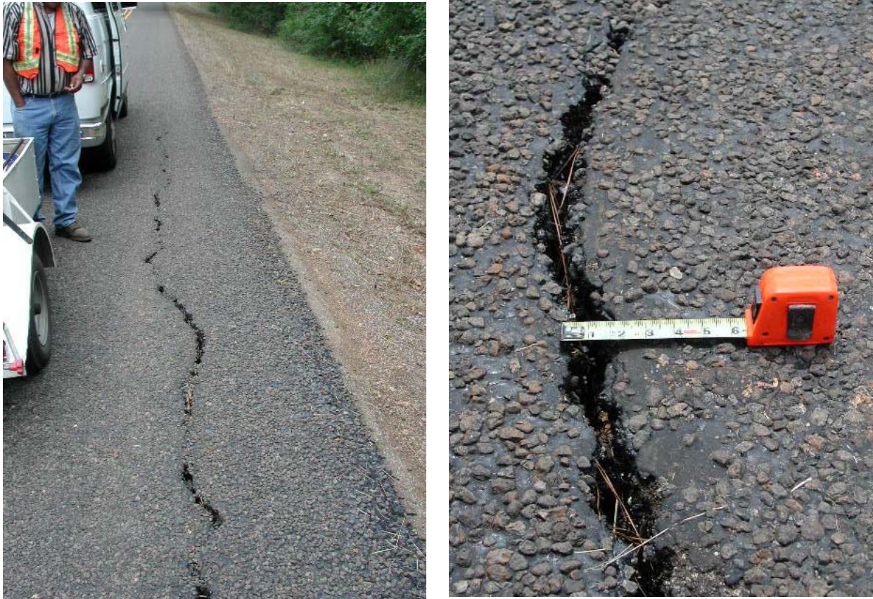
Figure 10. Core Location by Severe Crack on FM 2076 EB in Rehab Section.
