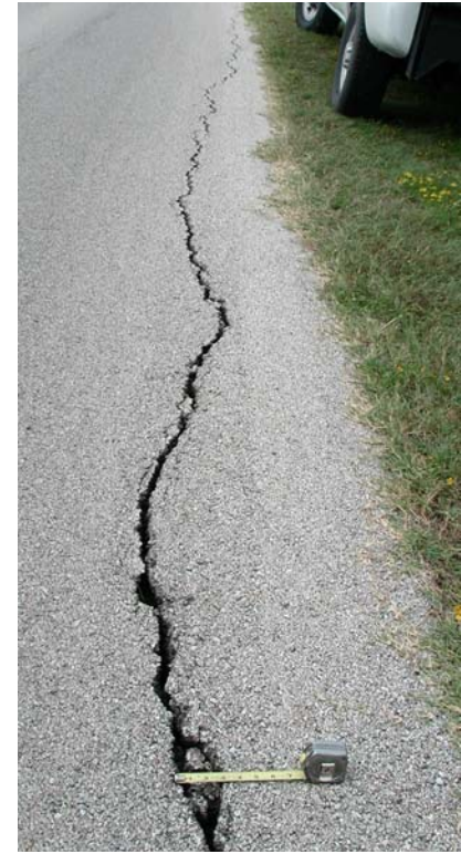
High Severity Longitudinal Cracking
