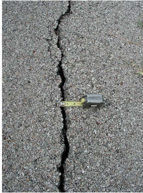
Medium Severity Longitudinal Cracking
