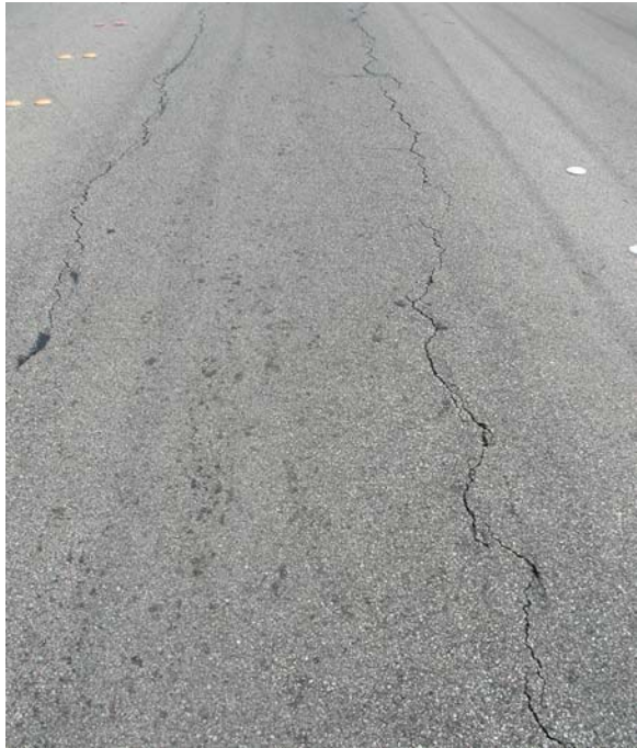
Low Severity Fatigue Cracking
