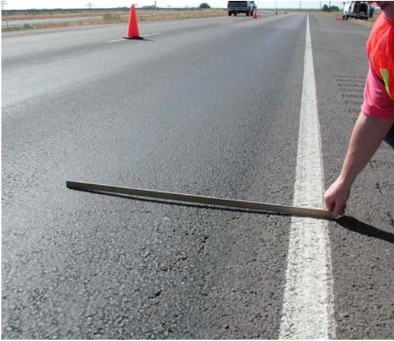
Low Severity Rutting
