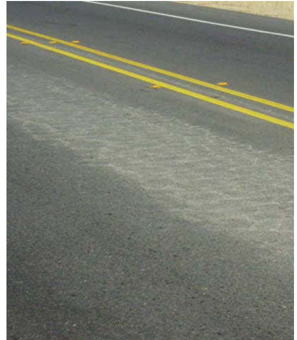
High Severity Fatigue Cracking
