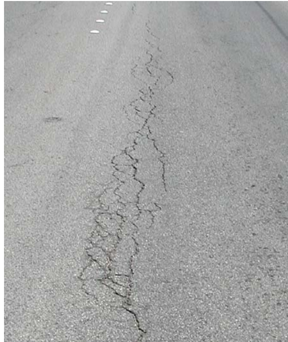
Medium Severity Fatigue Cracking
