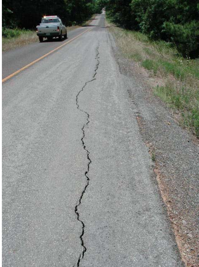
Figure 9. Severe Longitudinal Crack in FM 2076 WB Rehab Section.
