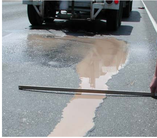
Medium Severity Rutting
