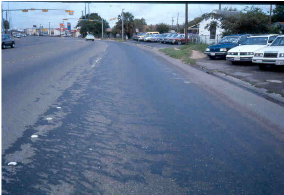
Figure 22. Severe Flushing From Underseal.
