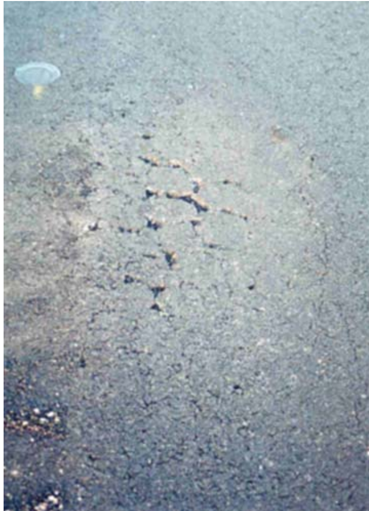
Figure 37. Cracking Distress on IH 20 Near Pecos.
