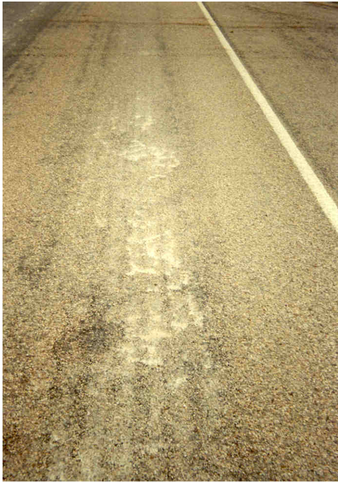
Figure 34. Alligator Cracking Distress on Loop 390 in Atlanta.
