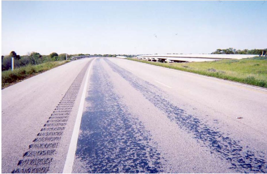
Figure 2-2. Excess Asphalt from Underseal Migrating Through to HMAC Surface.
