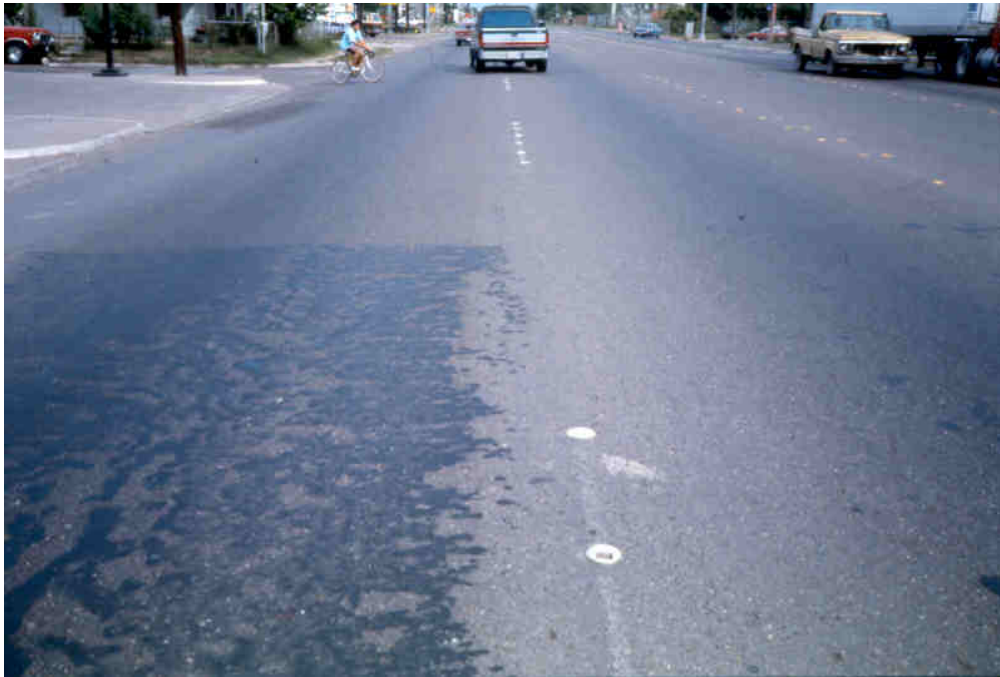
Figure 20. Underseal Test Section Bleeding Through to Surface.
