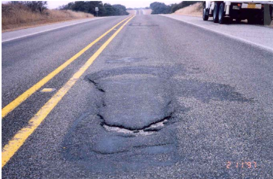
Figure 28. US 190 Pavement Failure.
