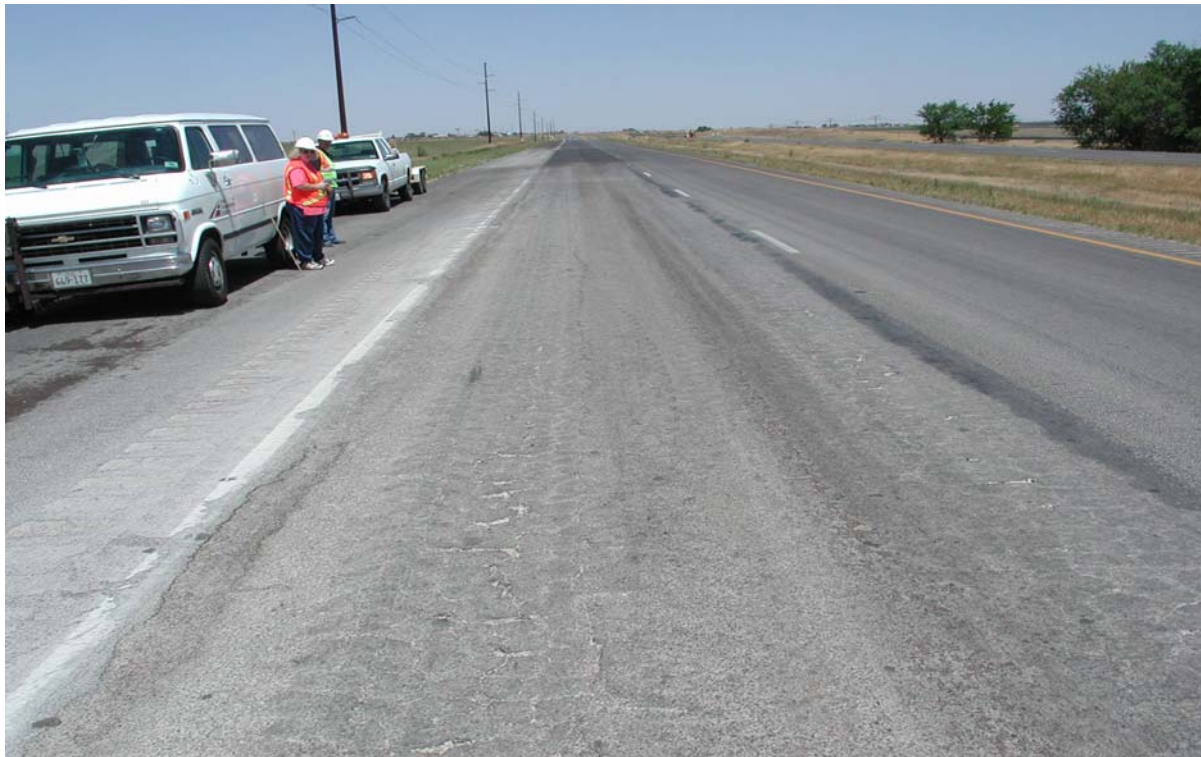
Figure 40. Damage on US 84 in West Texas.
