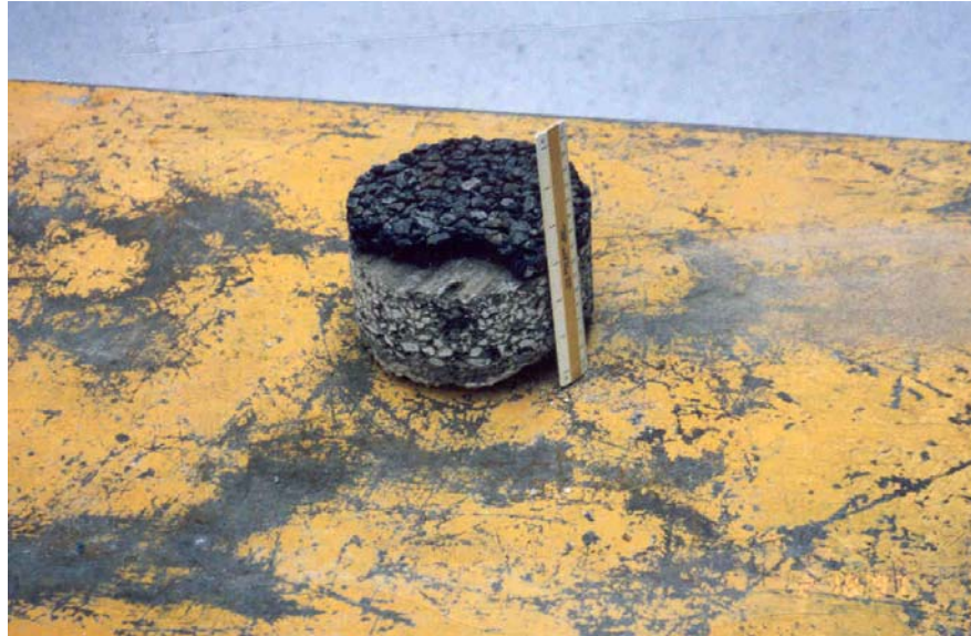
Figure 31. Pavement Cores Showing Debonded Overlay.
