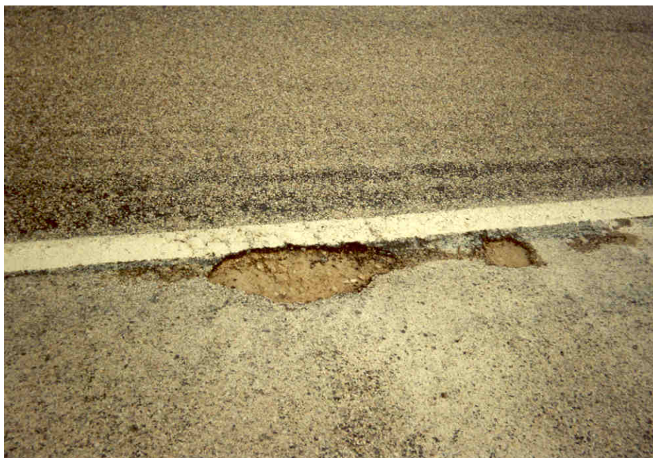
Figure 33. Delamination of One-Course Surface Treatment (Loop 390).
