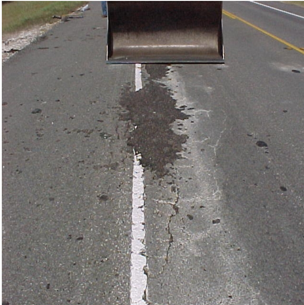
Figure 25. Distressed Area on SH 7.
