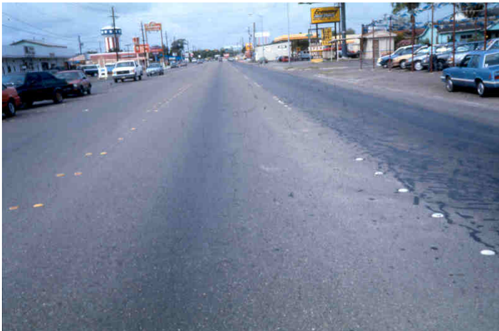
Figure 21. Inside Lane Test Sections Flushing Less Than Outside Lanes.
