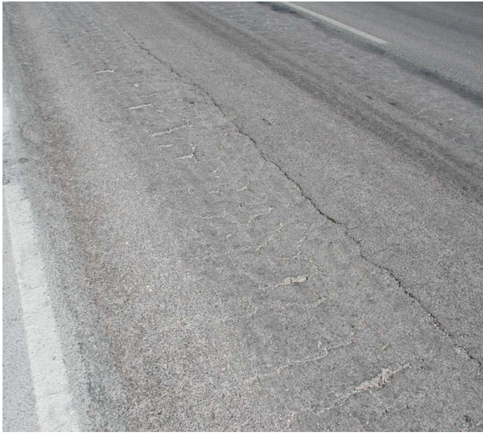
Figure 41. Close-Up of Damage on US 84.
