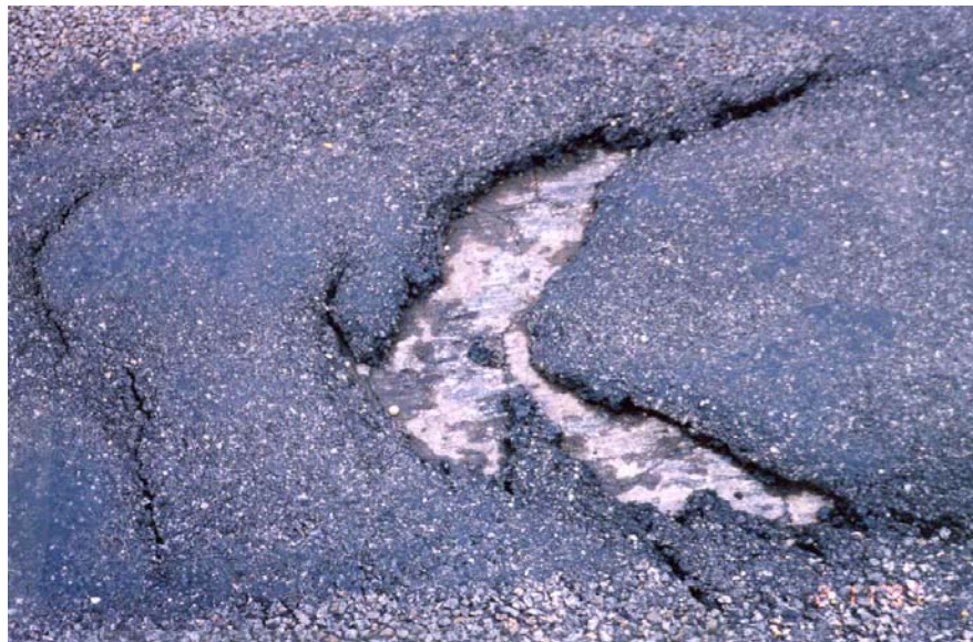
Figure 29. Close-Up of US 190 Pavement Failure.
