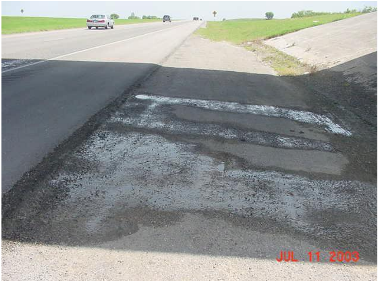
Figure 39. Moisture Seepage from IH 37 in Atascosa County.
