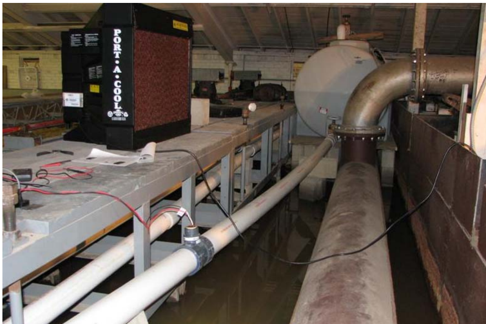
Figure 6.4. Upstream Reservoir and Water Tank.
