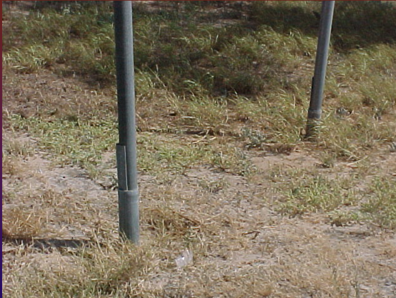
Ground stub too high
