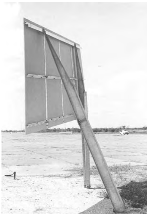
Figure 3-7: Rectangular slip base that performed as intended.
