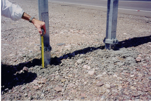
Figure 3-1: Stub heights should be less or equal to 4” to minimize the potential for vehicle snagging at the undercarriage. Each support has a specific stub height requirement – refer to the standard drawings for further detail.
