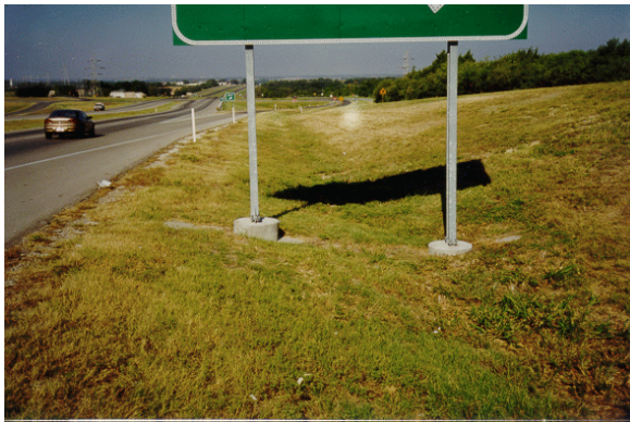
Figure 3-2: The grading of surrounding terrain should enable an errant vehicle to pass over any non-breakaway portion of the post installation. To ensure this, the AASHTO Roadside Design guide provides a recommendation as shown in Figure 3-3.
