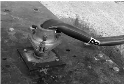
Figure 2-5: Slip Base did not activate
