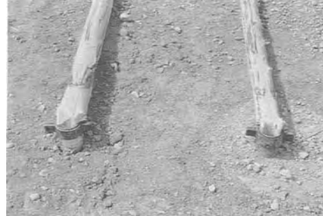
Figure 3-8: Fiberglass post socket system that did not perform as intended
