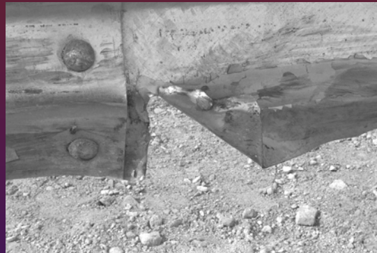
Partial tear in rail
