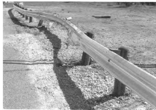
Figure 1-5: Guardrail with round wooden post that failed.
