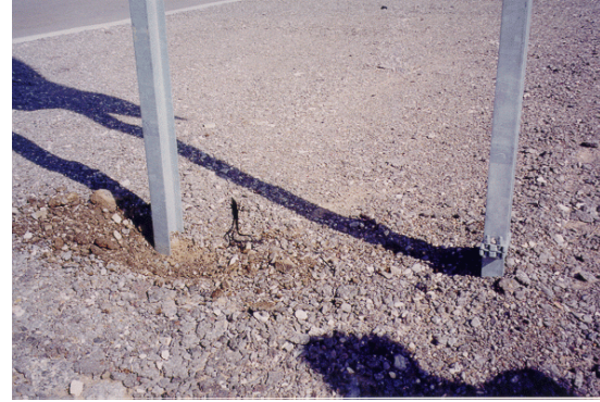
Figure 3-4: When breakaway sign bases are buried, additional force may be required to activate the breakaway base. Care should be taken during initial grading and maintenance activities.
