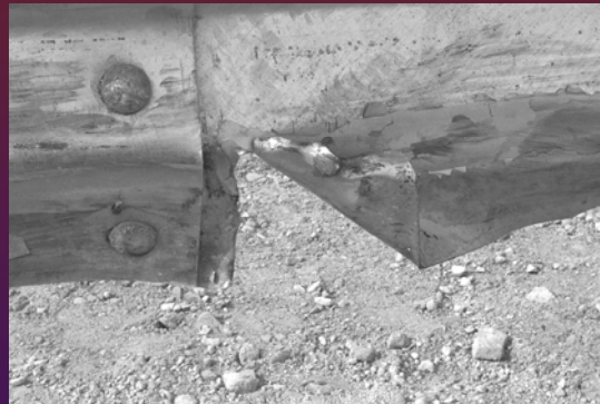
Partial tear in rail
