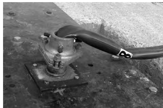
Figure 3-12: Slip Base did not activate
