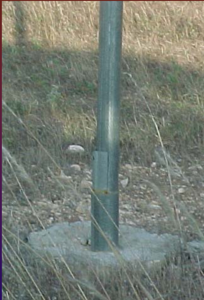
Stub too high
