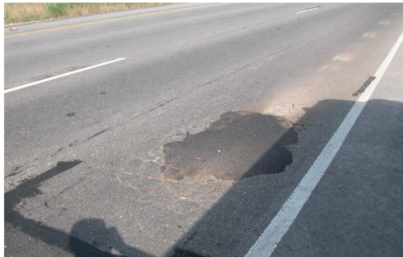
Figure 22. Rapid Deterioration to Structural Failure.
