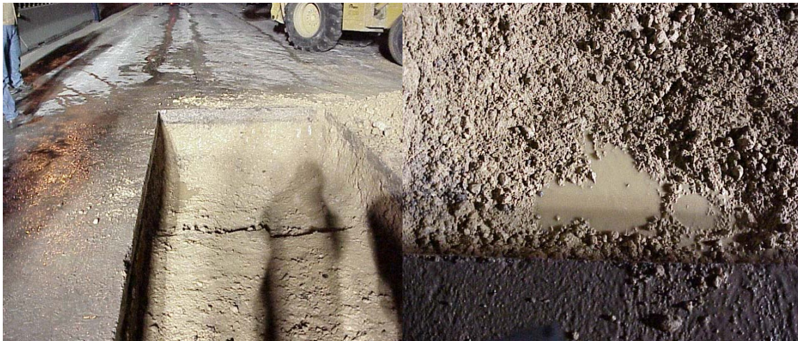
Figure 26. Trench in Failed Area of IH 35 (Chen, 2004).
