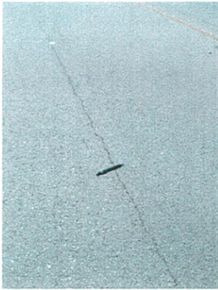
1. Typical mid-lane crack
