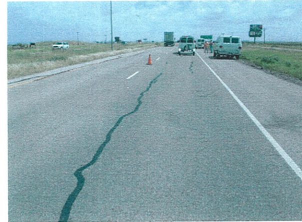
2. Longitudinal crack in left wheel path
