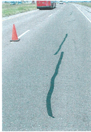
2. Typical sealed cracks
