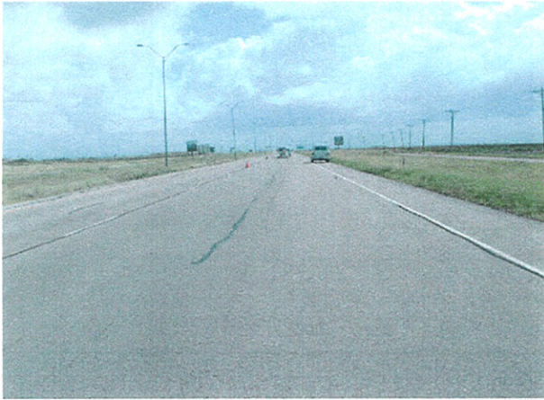
1. Typical sealed longitudinal cracks
