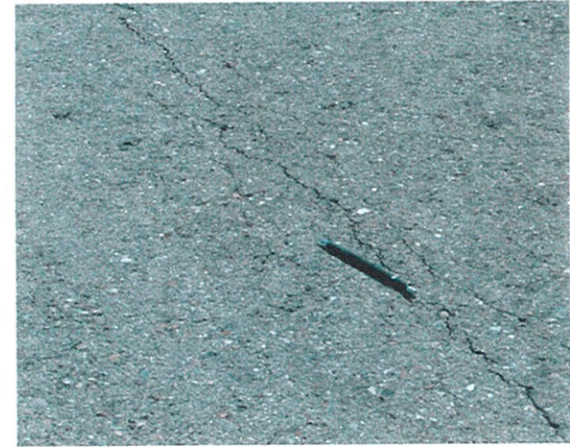
3. Typical unsealed cracks on shoulders
