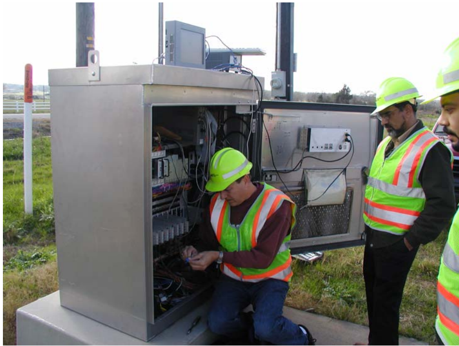
Figure 20. Researchers Installing the System in College Station.
