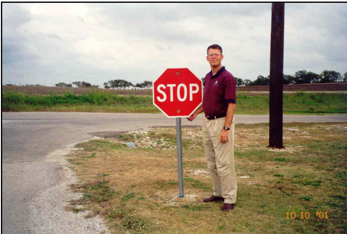
Figure 55. Sign on Elementary Site Mounted Several Feet below the Standard Height.
