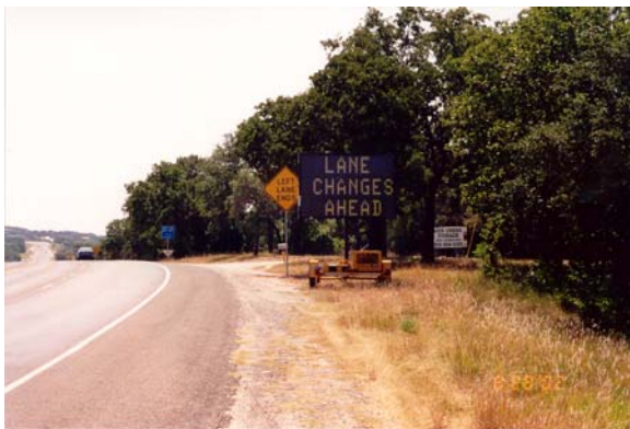
Figure 4-8. Changeable Message Sign and Sign Showing Changes to Roadway.
