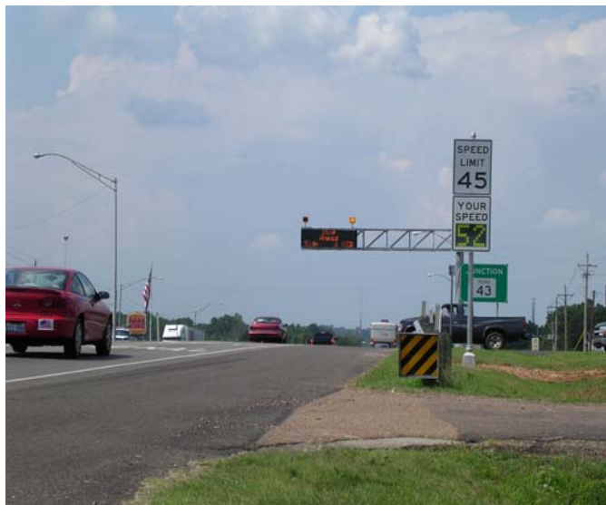
b. Cantilevered electronic matrix warning sign located in Marshall, Texas.
