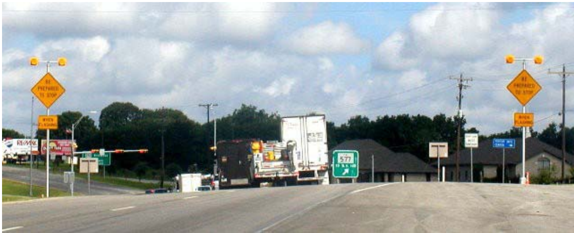
Figure 19. Westbound US 290 Approach in Brenham after AWECS Installed.
