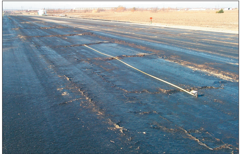
Figure 1. Vertical Heaves Generated during Construction of US 67 near Midlothian.
