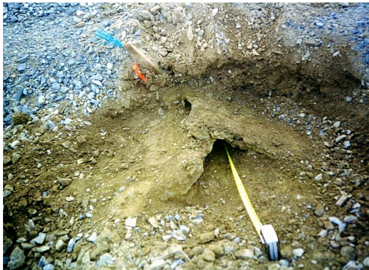
Figure 15. Trench Cut along Heaved Section of US 82.
