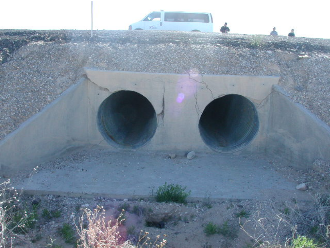
Figure 31. Expansion of Cement-Treated Backfill on SH 54 North of Van Horn.
