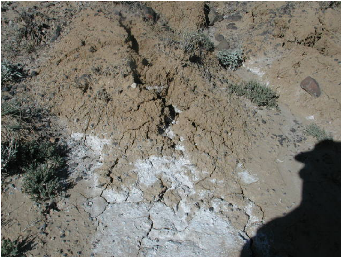
Figure 28. Efflorescence Observed on SH 118 South of Alpine.
