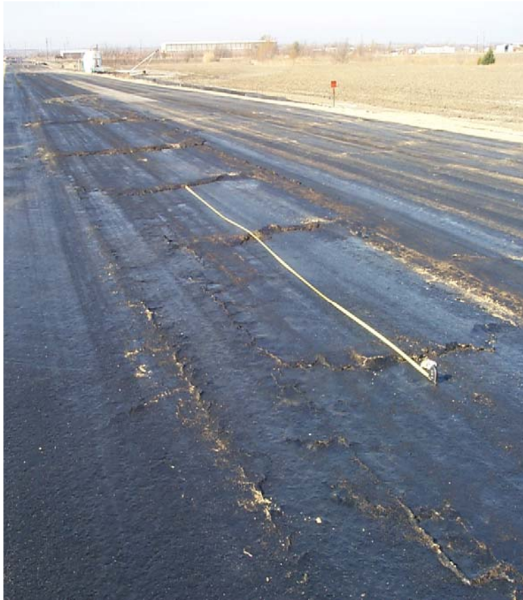
Figure 18. Vertical Heaves of Lime-Stabilized Subgrade on US 67 in Ellis County.
