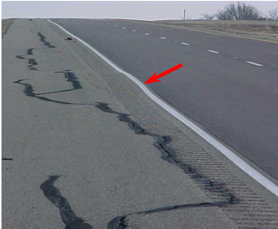
Figure 25. Longitudinal Cracks on Shoulder and Swell (solid white line marking the shoulder) near Baylor Creek on US 287. (Image courtesy of Zhiming Si)
