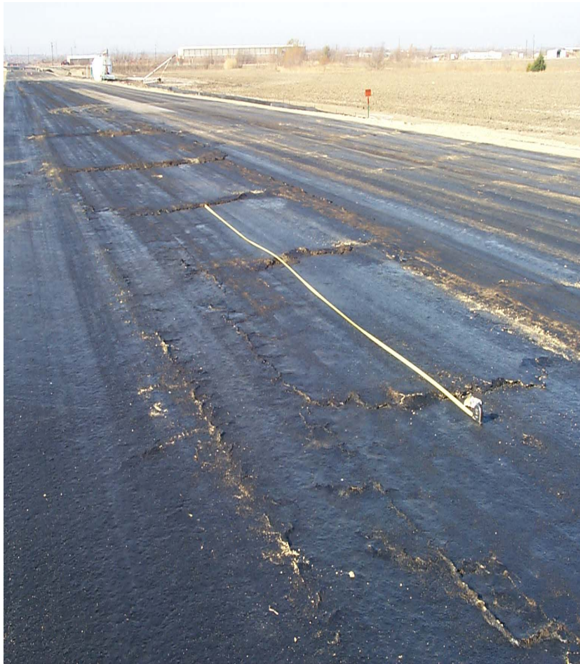
Figure 1. Vertical Heaves Generated during Construction of U.S. 67 near Midlothian.
