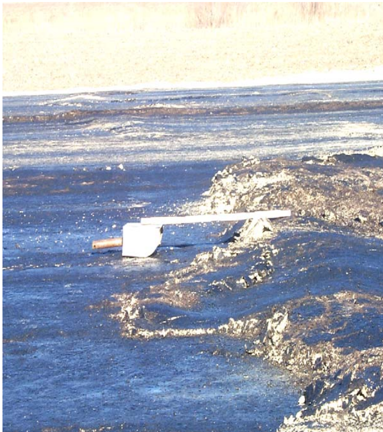
Figure 1. Vertical Heaves Generated during Construction of U.S. 67 near Midlothian.
