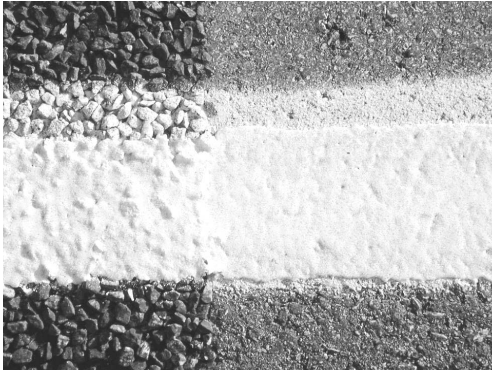
Figure 16. Thermoplastic Marking on HMA vs. Sealcoat.
