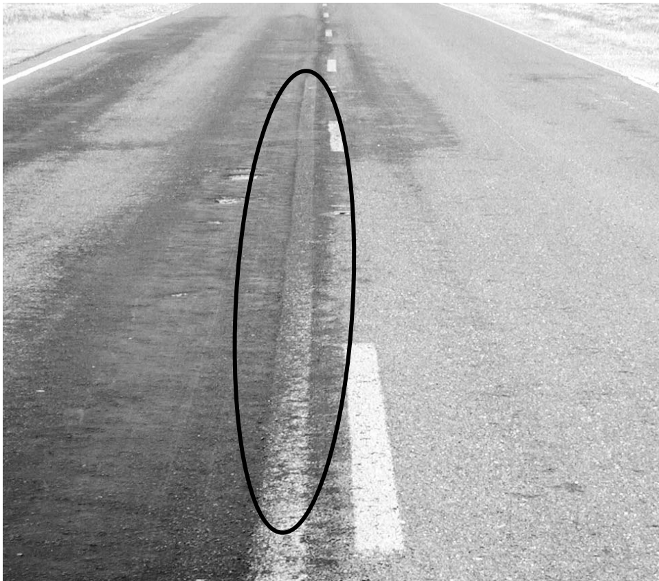
Figure 15. Asphalt Tracked onto Markings.
