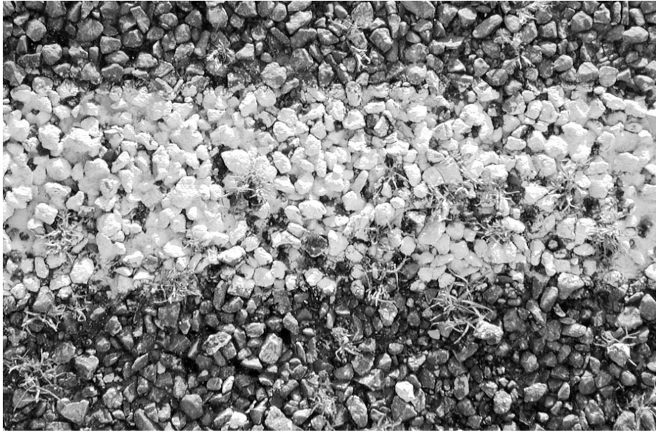
Figure 13. Pavement Marking on Sealcoat with Aggregate Roll and Pop-Out.
