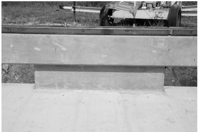
Figure B-2. Test Article/Installation before Test 441382-2
