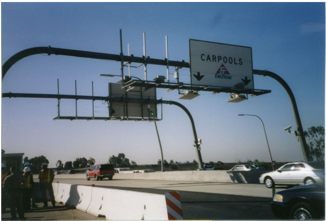
Figure 3. Example of Signage and ETC for a Special (Discount) Lane for HOVs.
