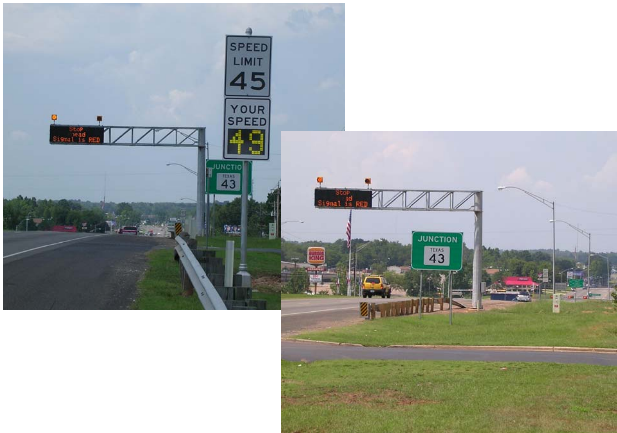
Figure 13. Dynamic Message Sign as Advance Warning of a Signalized Intersection near a Vertical Curve.
