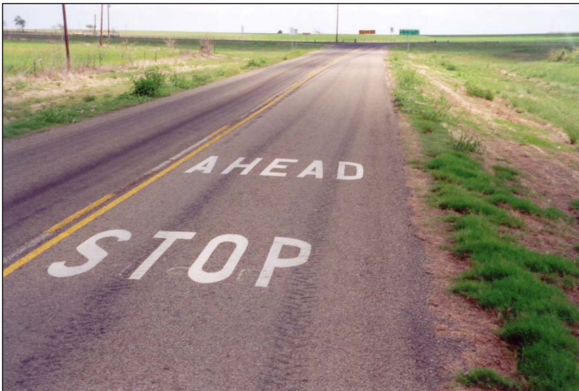
Figure 5-11. Advance Warning Pavement Markings on Intersection Approach.
