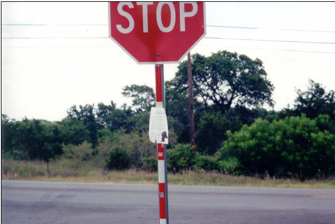
Figure 5-3. Reflective Strips on STOP Sign Post.
