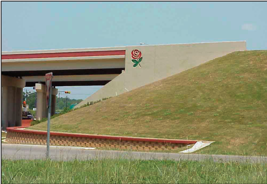
Figure 3. Form-Liner Finishes Can Be Used to Create Highly Detailed Murals on Retaining Walls.
