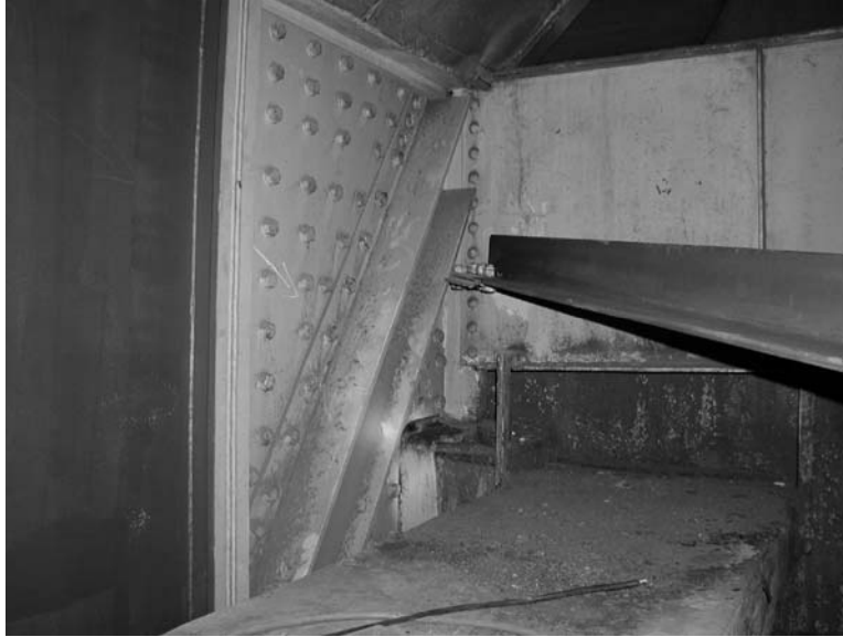
Figure 109. Rib and Lateral Brace Used to Reduce Out-of-Plane Bending.
