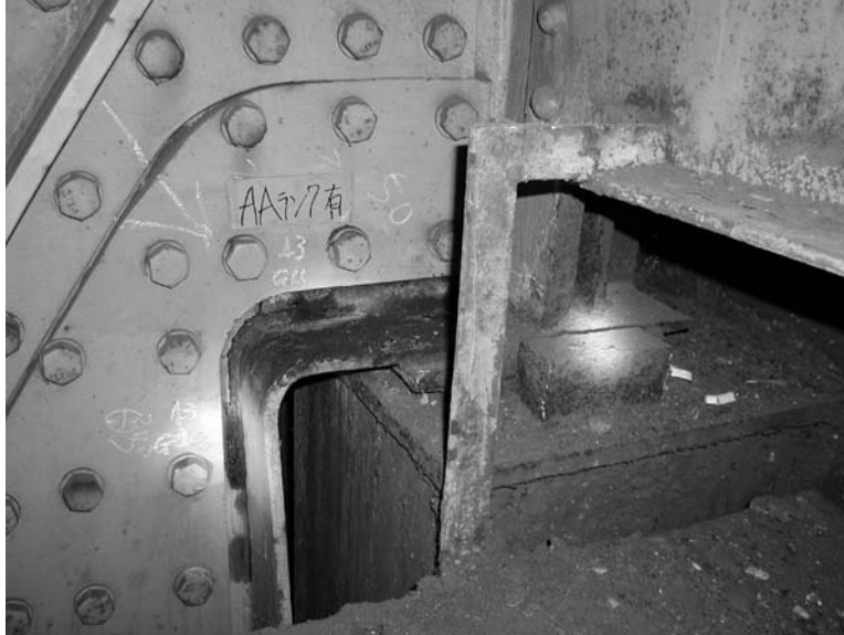
Figure 110. Fatigue Crack That Continued to Propagate after Retrofit.
