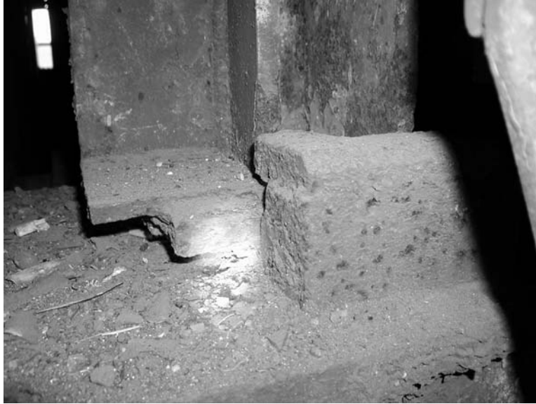
Figure 106. Corrosion of Beam Seat.
