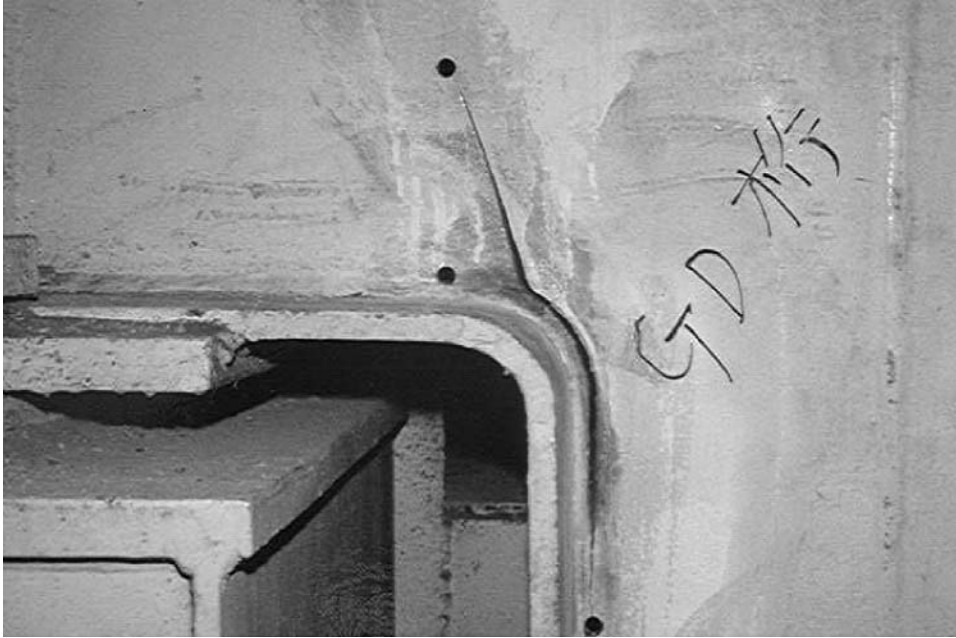
Figure 100. Fatigue Cracks in 90-Degree Rounded Detail in Japan.
