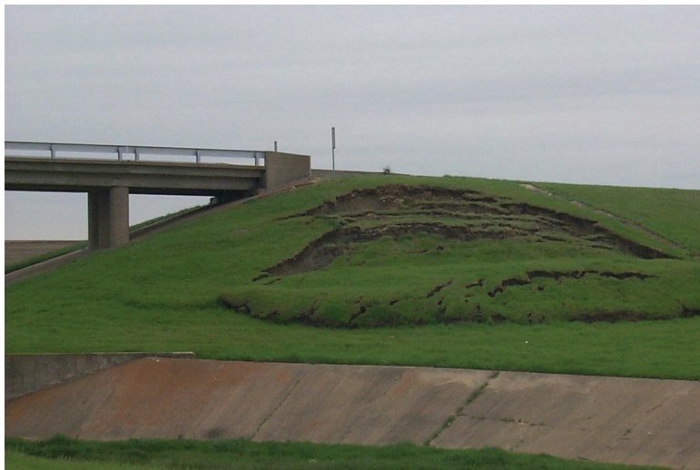
Slope failure like that shown here illustrates the need to investigate long-term strength of high-PI clays.
