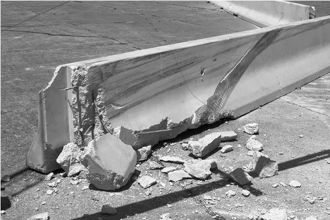
Figure 12. Grid-Slot Barrier with U-bar Connector After Crash Test.
