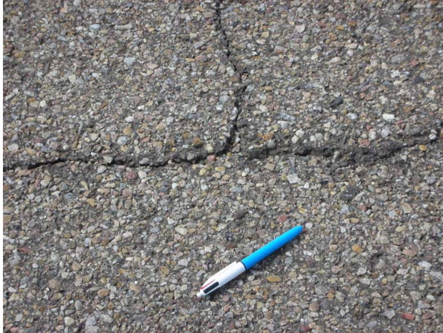
Figure 3-10. Reflective Crack on Amarillo Test Pavement in 2007.
