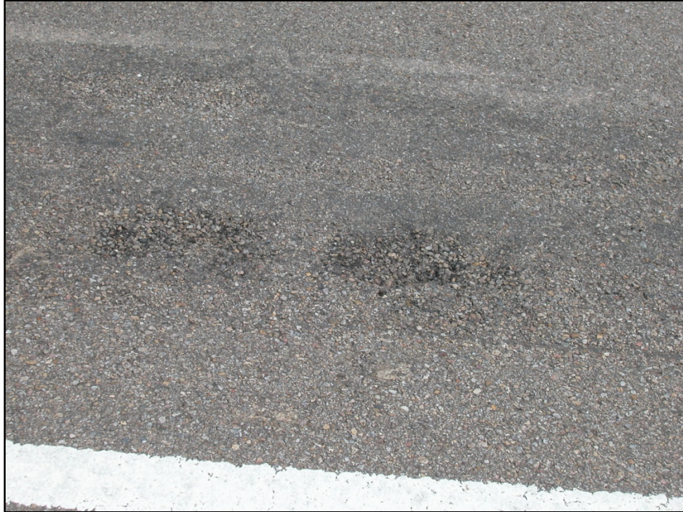
Figure 3-12. Raveling Observed in the PaveTrac Section in 2004.
