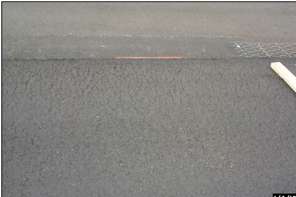
Figure 17. Checking (or Crazing) Observed During Portions of Overlay Paving.
