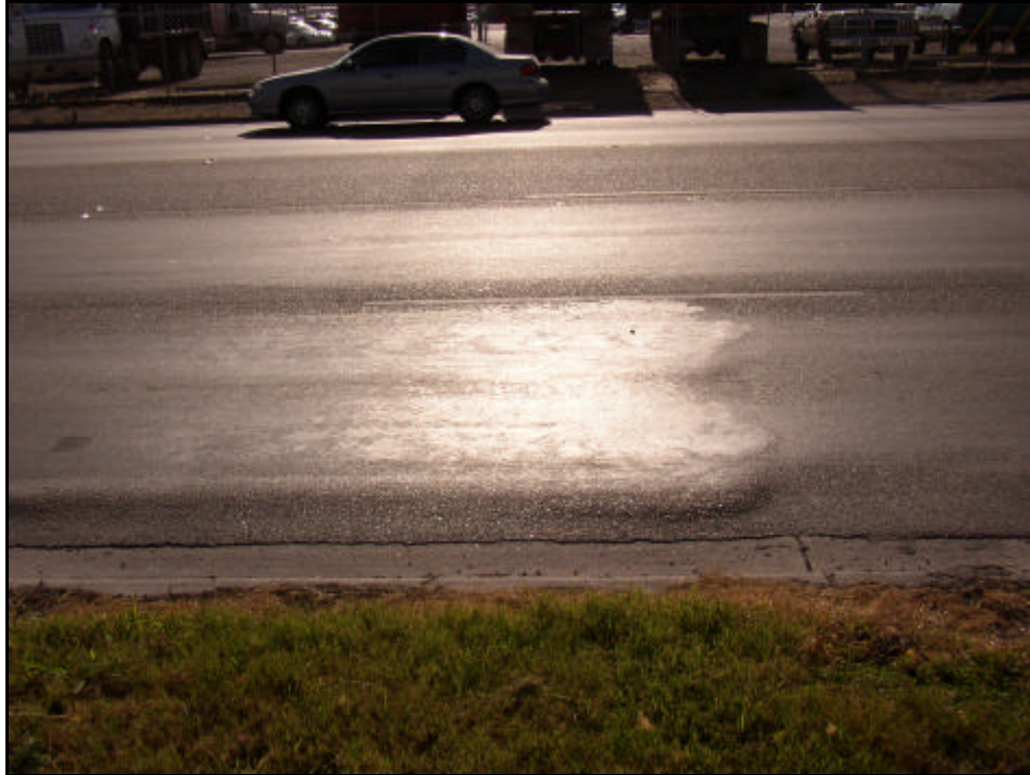
Figure 5. Shoving with Flushing at an Intersection Approach in McAllen.
