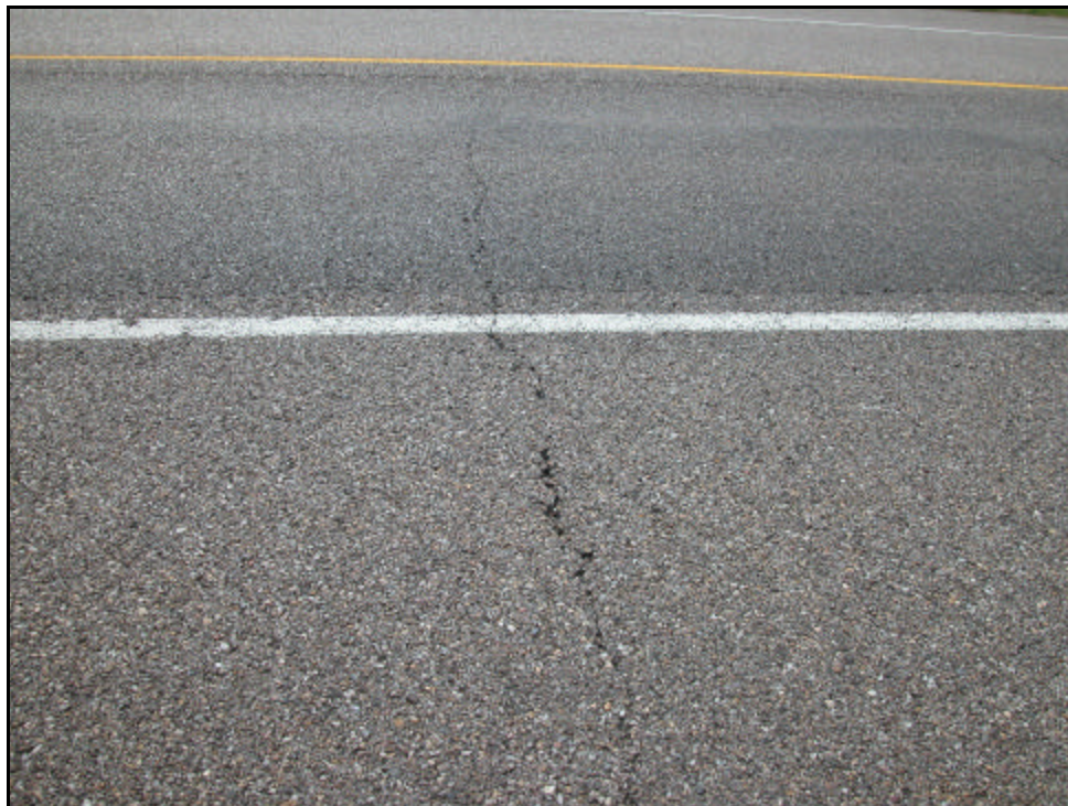
Figure 20. A Transverse Crack in PFC with Leveling Course Test Section.
