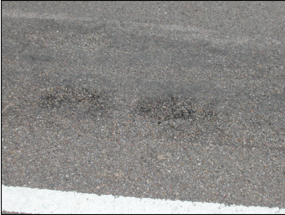
Figure 19. Raveling Observed in the PaveTrac Section in 2004.
