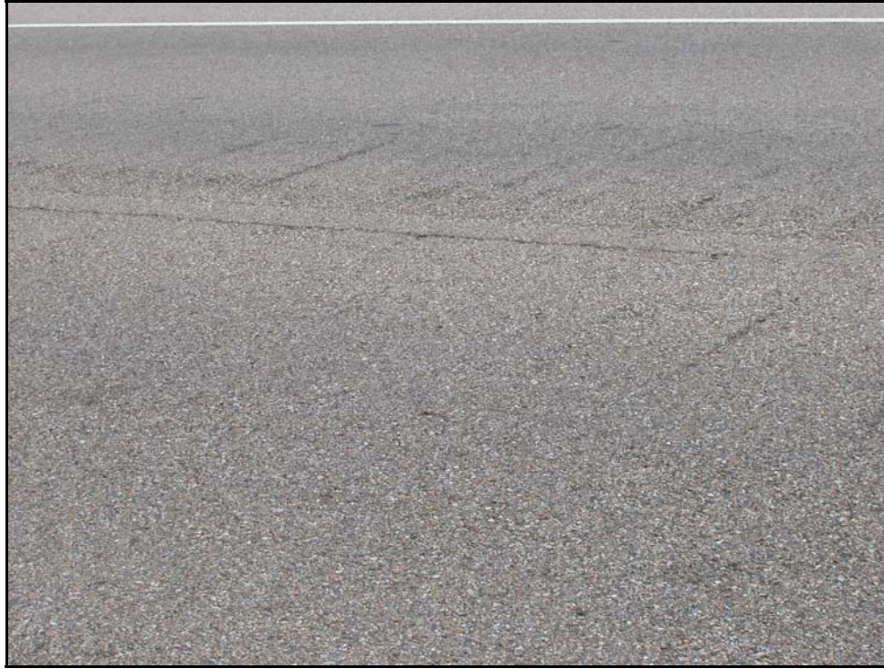
Figure 21. Short Parallel Transverse Cracks Radiating from the Centerline of the PaveTrac Section.
