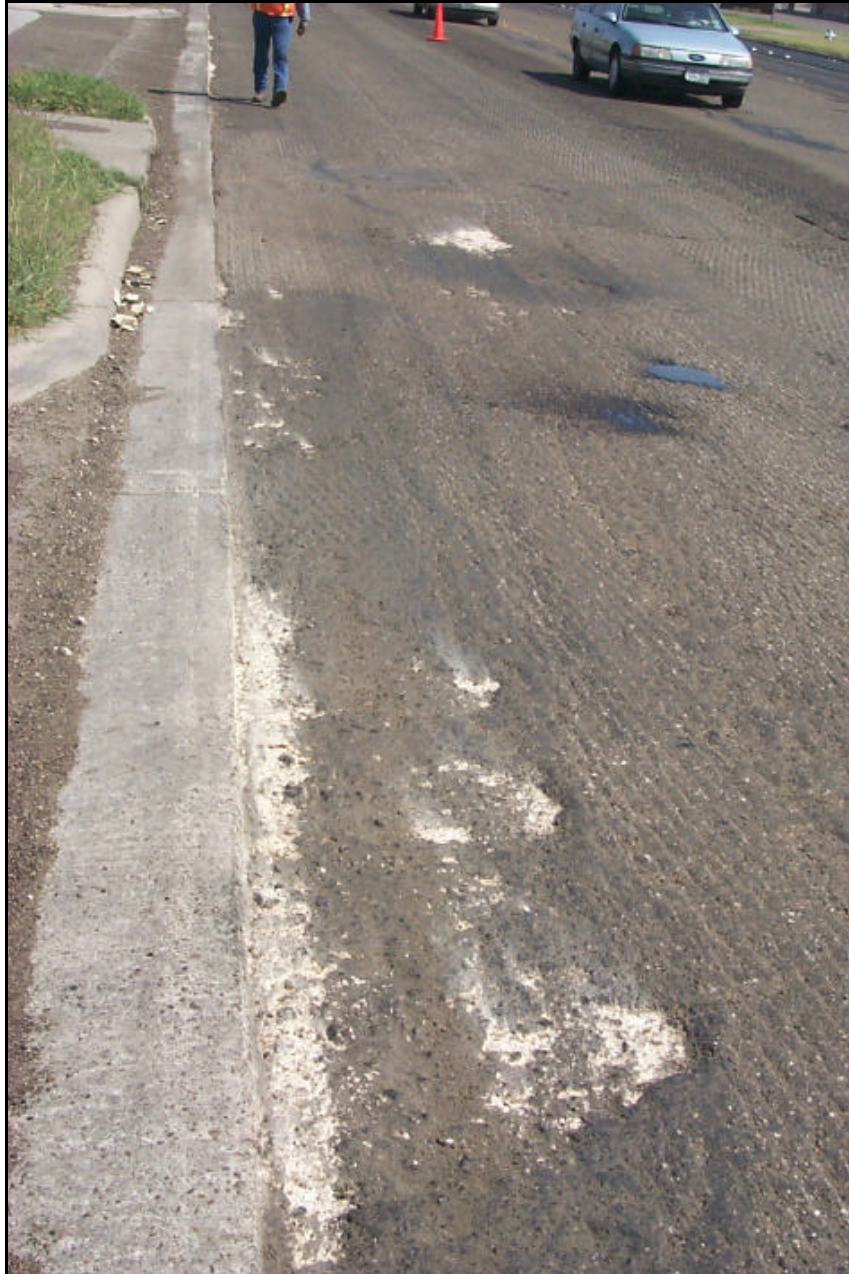
Figure 3. View of Exposed Base due to Milling Operation.
