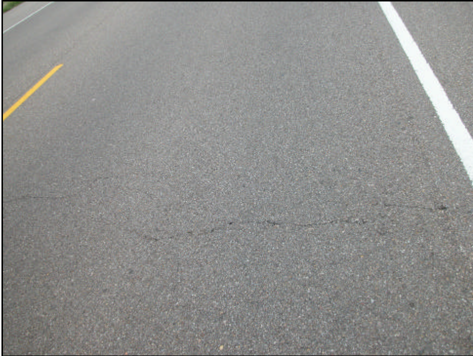
Figure 18. Transverse Crack Observed in 2004 in Hot-In-Place Recycled Section.
