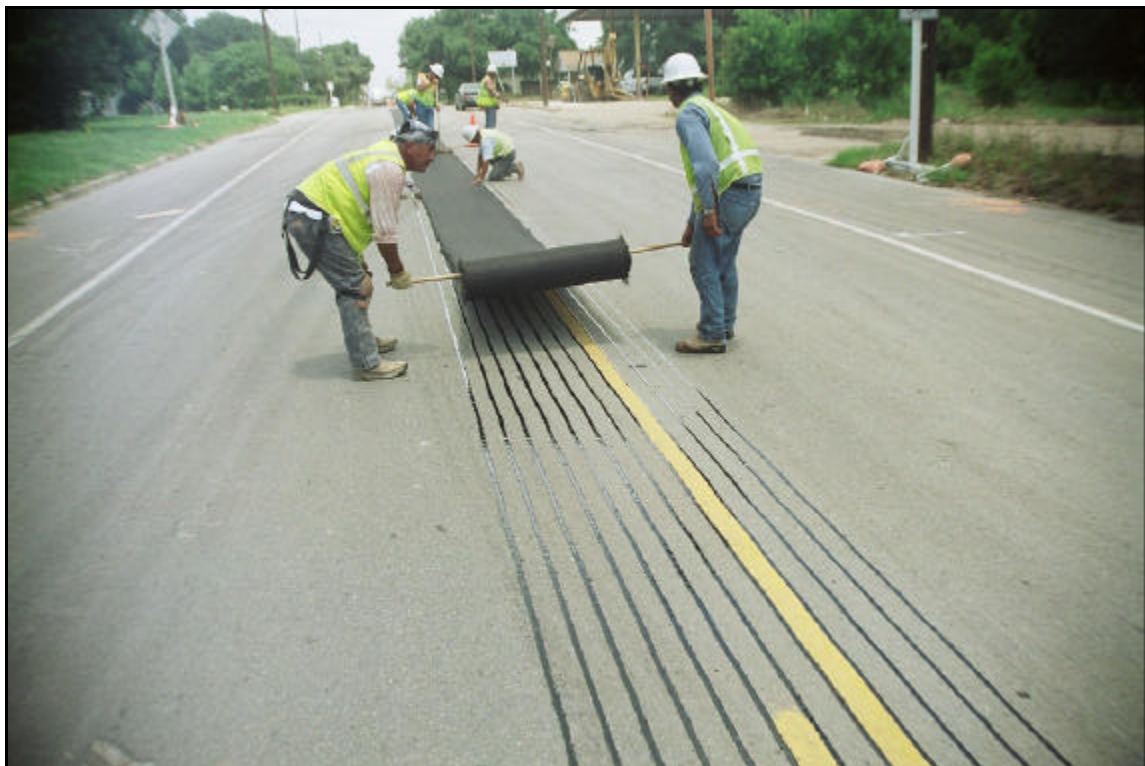
Figure 9. Example of Dribbled, Insufficient Asphalt Tack.
