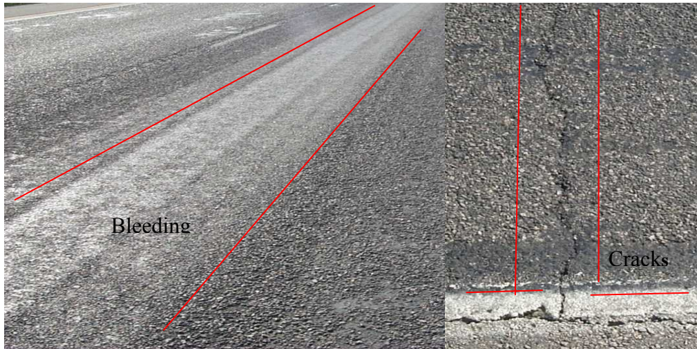
Figure 25. Inadequate Performance on HS1 – Pictorial.
