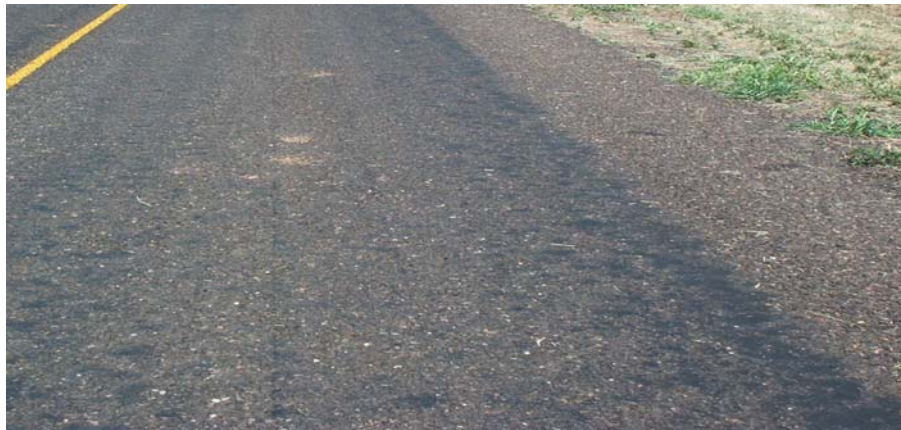
Figure 23. Inadequate Performance on HS39 – Pictorial.
