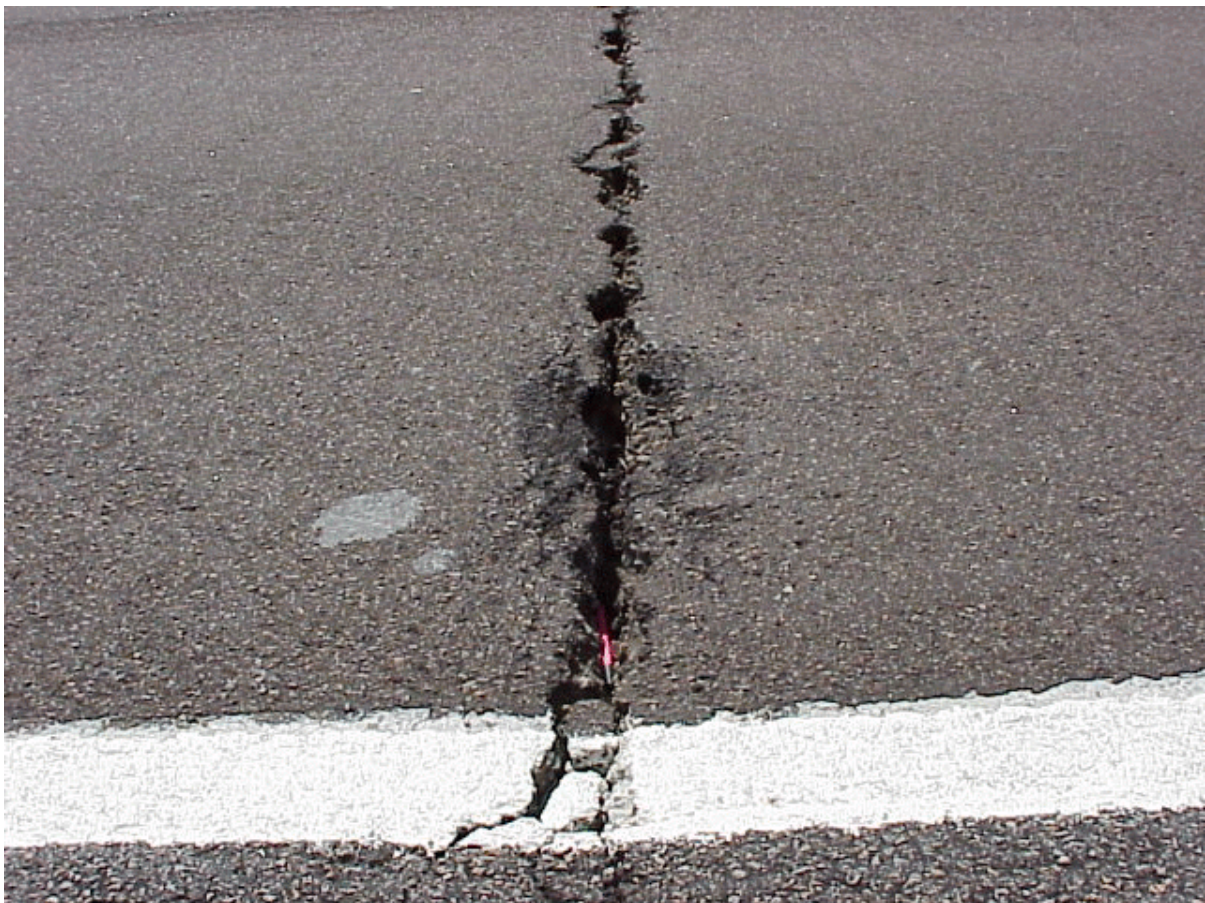
Figure 20. Photo of Severe Transverse Cracking along the I-20 Project.
