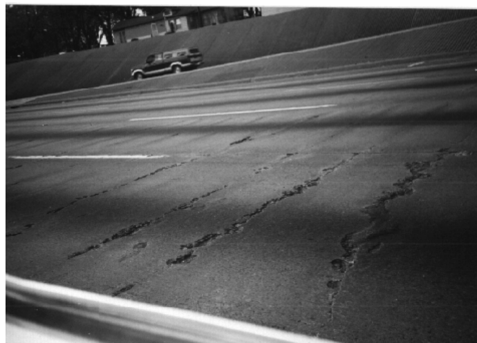
Figure 4. Spalling in CRC Pavement (13).
