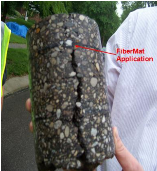
Figure 4. FiberMat slows down the cracks
