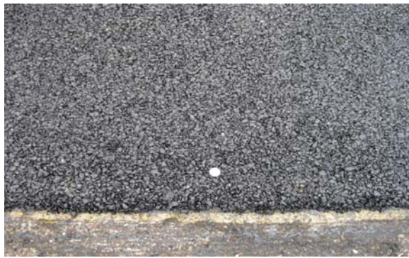
Finished RHMA-O warm mix overlay in Route 94, San Diego, CA (TRB 11-0445 pg. 14)
