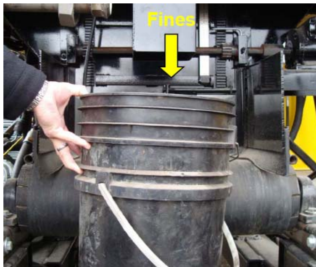
Dry Additive Calibration
