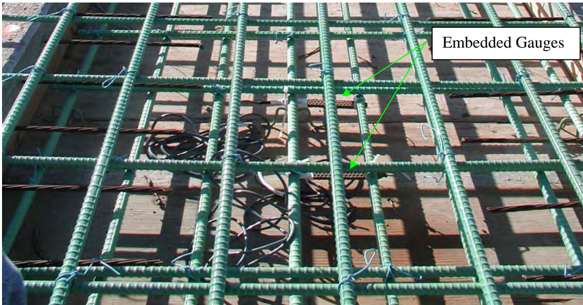
Figure 3.10 Embedded Gauges in the Controlled Joint Between Spans 1 and 2
