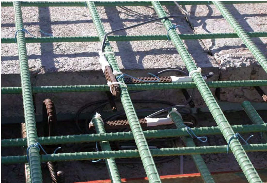
Figure 3.4. Embedded Concrete Strain Gauges Over an Interior Beam
