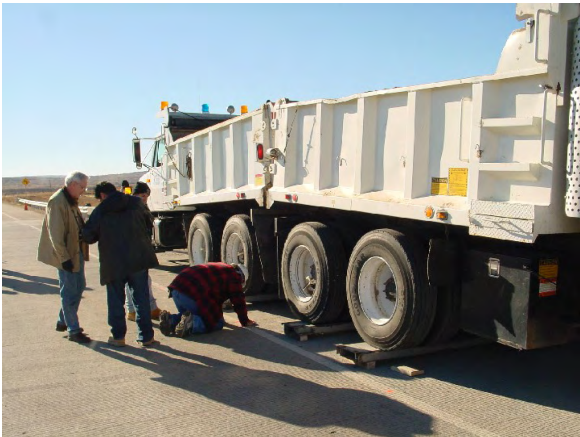
Figure 4.3 Crack Measuring with TxDOT Dump Trucks in a Back-to-back Load Case Photograph: Courtesy of Alvin Gutierrez, FHWA
