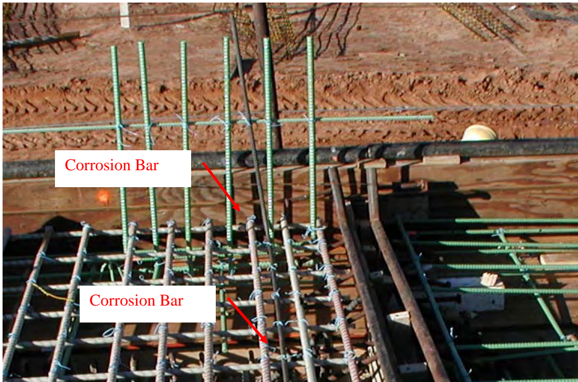
Figure 3.13 Corrosion Bar at the Sealed Expansion Joint (Discontinuous End) of Span 6, Phase I
