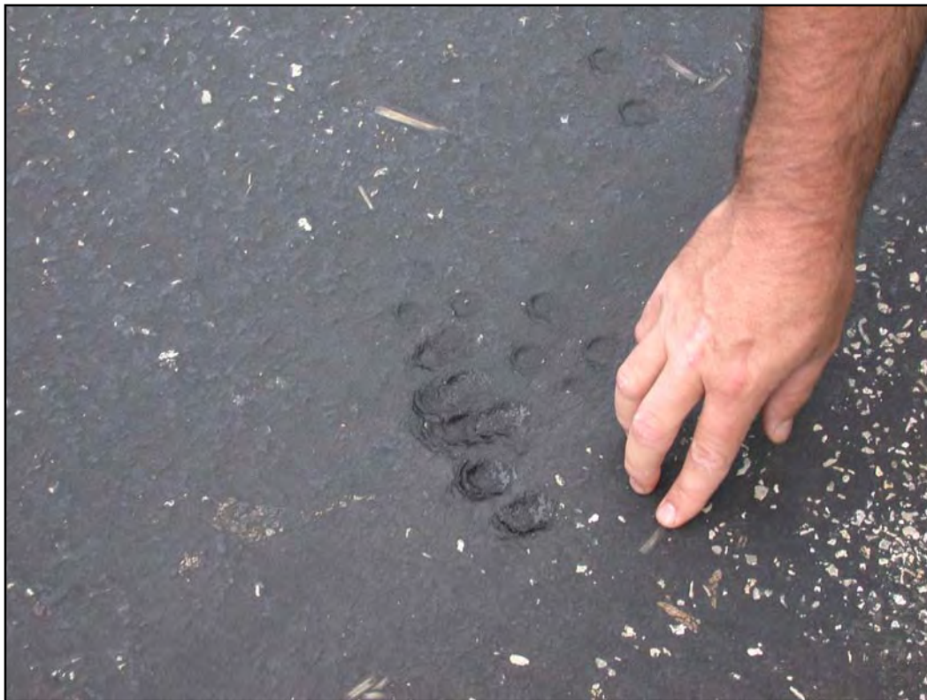
Figure 4.4 Soft Pavement (Flushing) Resulting From High Temperature/Humidity
