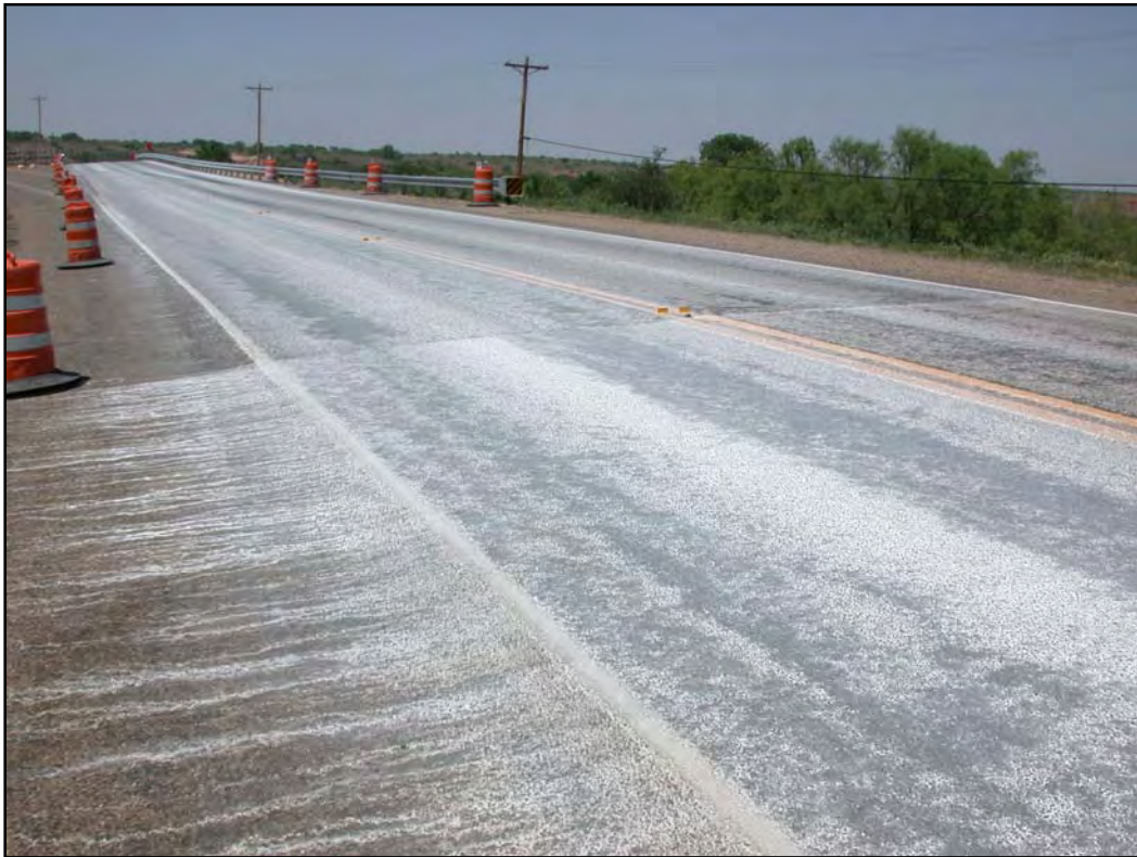
Figure 6.12 The Lime Application Rate Should Achieve Good Splatter (Dosage) of Lime Water Solution on the Affected Pavement Surface
