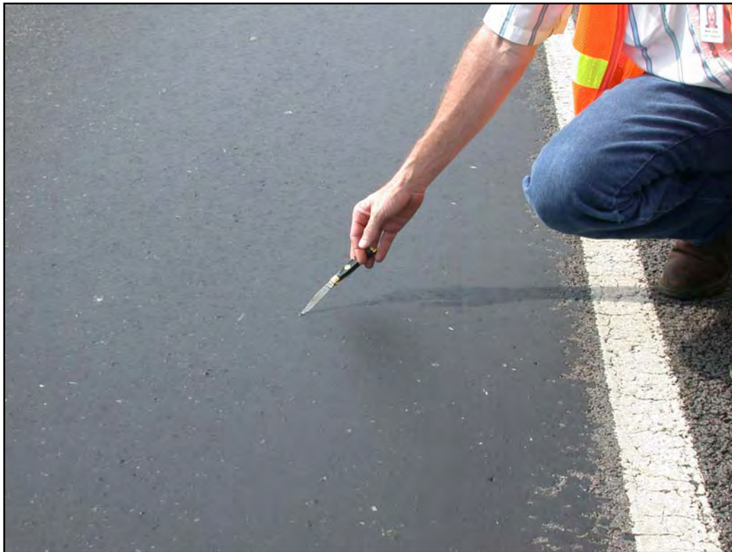
Figure 3.5 Heavily Flushed Pavement
