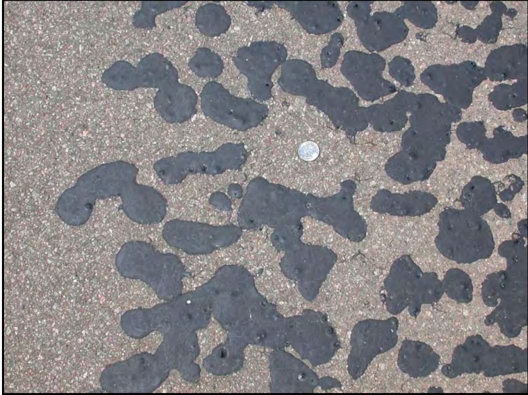
Figure 7.5 Excess Asphalt from Flushed Pavement Can Work Its Way Through Microsurfacing
