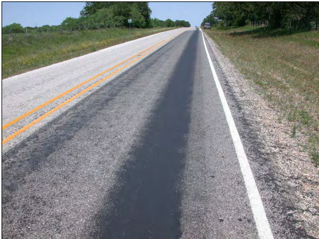
Figure 4.1 Flushing in Wheel Paths
