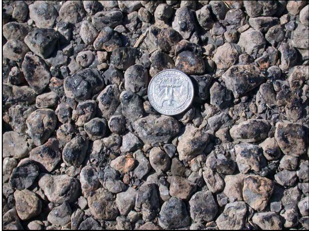
Figure 8.3 The Racked-In Seal Involves a Light Application of Small Size Aggregate (Scatter Coat) Over a Traditional Coarser Aggregate Seal Coat
