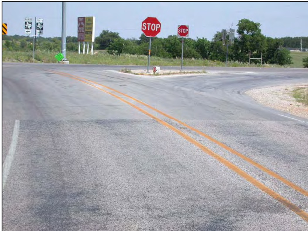
Figure 8.1 Use of Hot Mix Asphalt at an Intersection Largely Depends on Economic Considerations Including Life Cycle Costs
