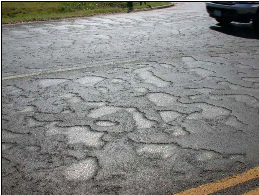
Figure 4.3 Pavement Distress Caused by Starting/Stopping and Turning Maneuvers
