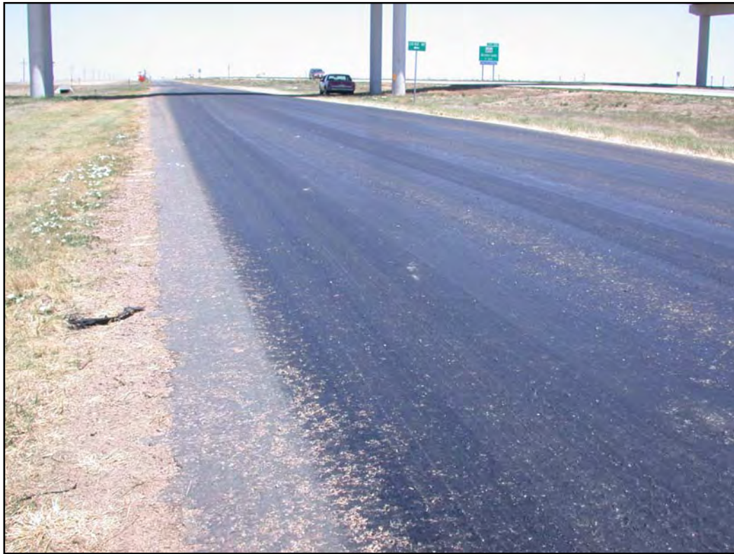
Figure 3.2 Bleeding Asphalt Caused by Excessive, Heavy Truck Traffic and Hot Weather
