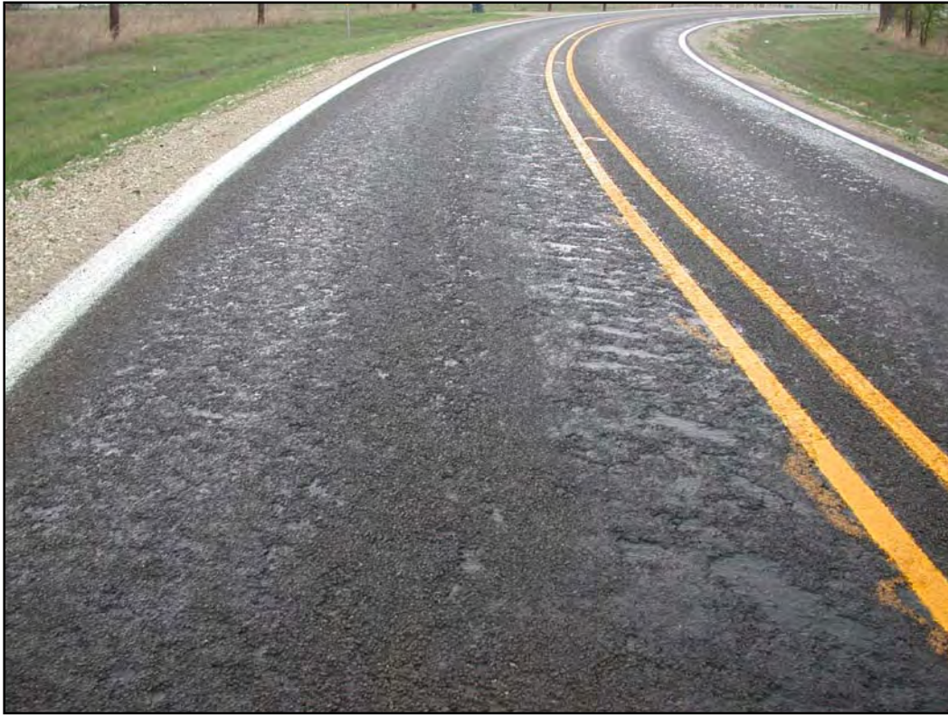
Figure 6.15 Removal and Replacement May Be Necessary When a Fresh Seal Coat Totally Fails
