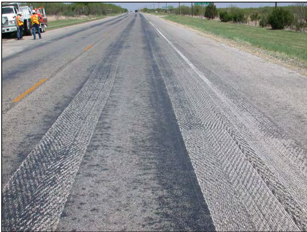
Figure 7.2 Cold Milling Yields a Grooved Surface Texture Along the Longitudinal Axis of the Roadway
