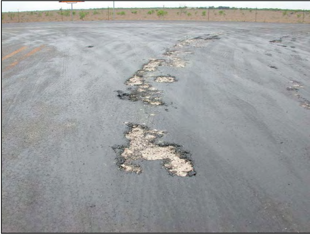
Figure 3.3 Pavement Damage – Picking Up of Seal Coat – Caused by Bleeding
