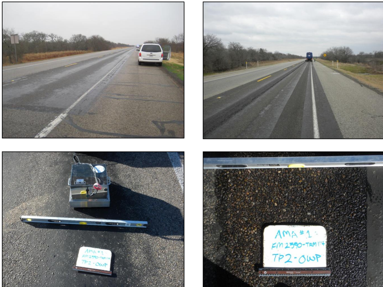
FIGURE 1.2 Pavement surface before treatment (left), and after treatment (right) using the UHP water cutter
