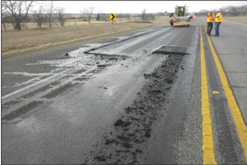
FIGURE 4.5. Flushed asphalt removed from the treatment operation left on the road when vacuum suction pump was turned off
