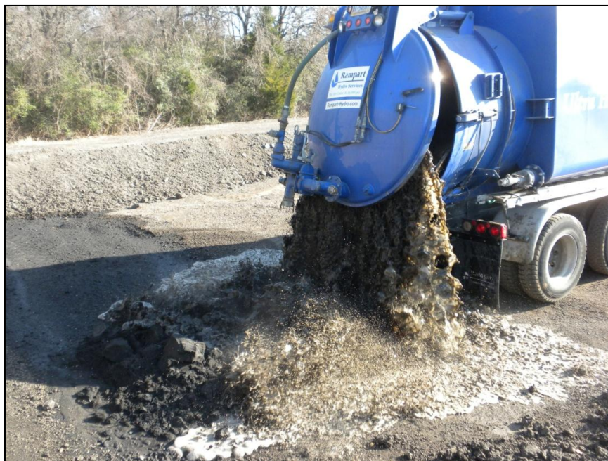
FIGURE 2.5. Debris tank and dump, Rampart BlasterVac truck
