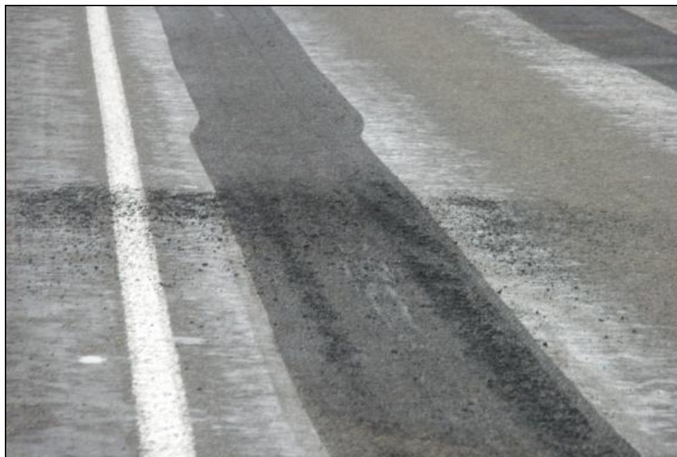
FIGURE 4.6. Traces of removed asphalt left on treatment path
