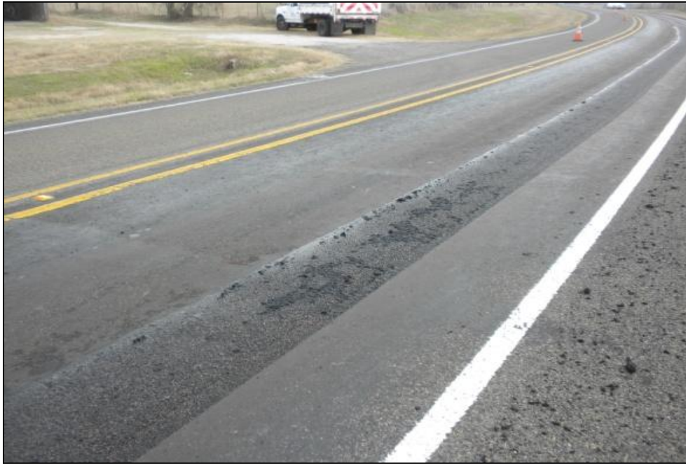
FIGURE 4.8. Treated wheel patch showing small amounts of asphalt not vacuumed and then pressed back into the lane by tires of the water cutter truck – this picture also shows the sharp edge sometimes left by the treatment at the edge of the strip
