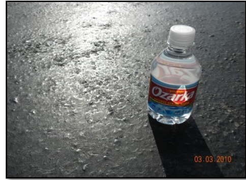
(b) Heavily flushed seal coat, pre-treatment
