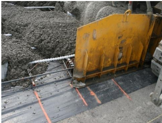
Figure 2.4 Longitudinal rebar placed to correct the problems of bars being pushed by concrete
