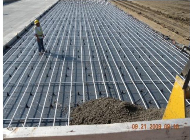
Figure 2.5 Longitudinal rebar placed at both sides and in the middle of the slab
