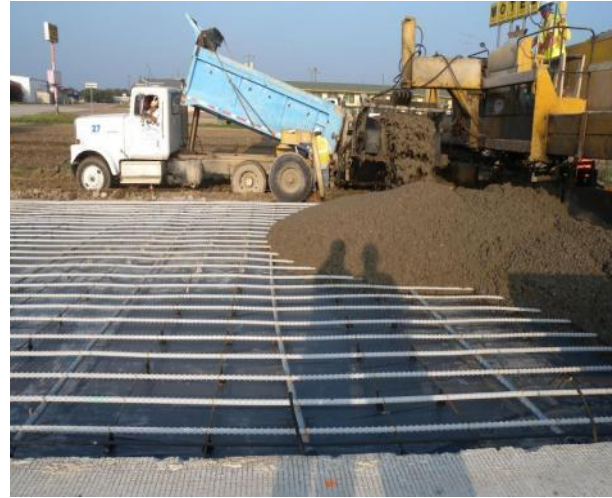
Figure 2.7 Transverse post-tensioning bar being bent due to concrete pressure
