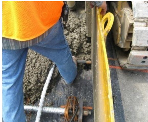
Figure 2.3 Contractor trying to hold transverse bars in place
