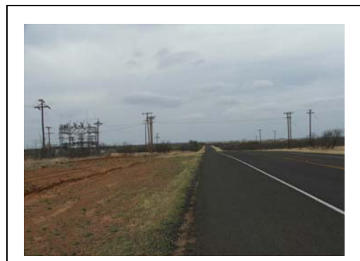
Figure 1.2 2183 kV transmission line, sub-station and 12.5 kV distribution line crossing a state highway
