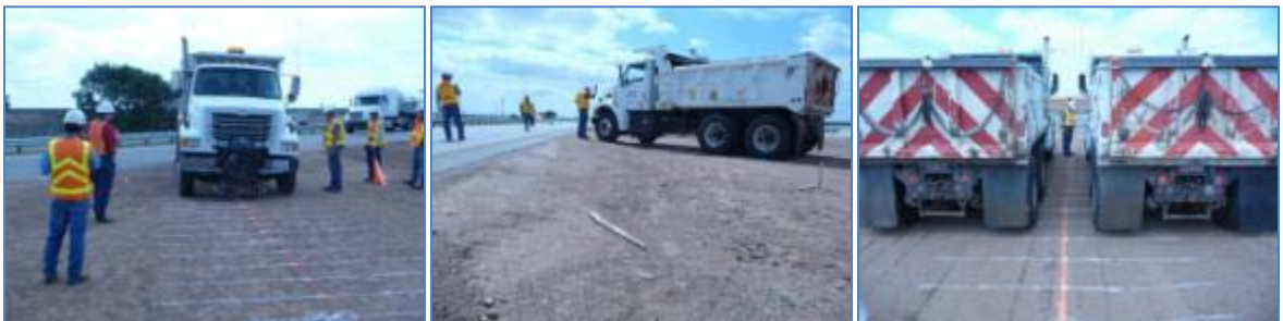
FIGURE 6.3. LIVE LOAD CONFIGURATIONS: A) TRUCK STRADDLING GAGE LINE B) WHEEL ON GAGE LINE C) 2 TRUCKS STRADDLING GAGE LINE.
