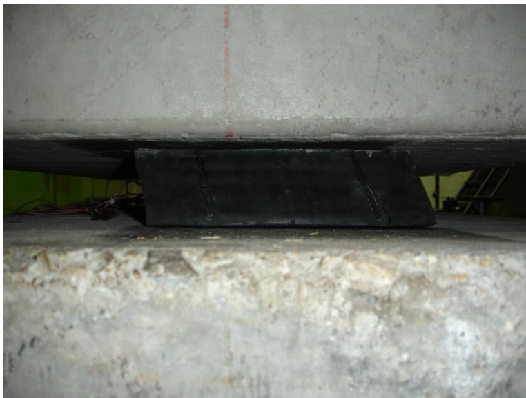
Figure 5.54 – Bearing Corner Undergoing Curling
