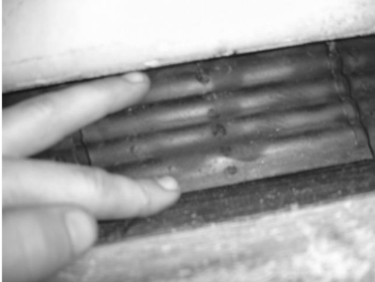
Figure 5.75 – Tension Debonding at Shims
