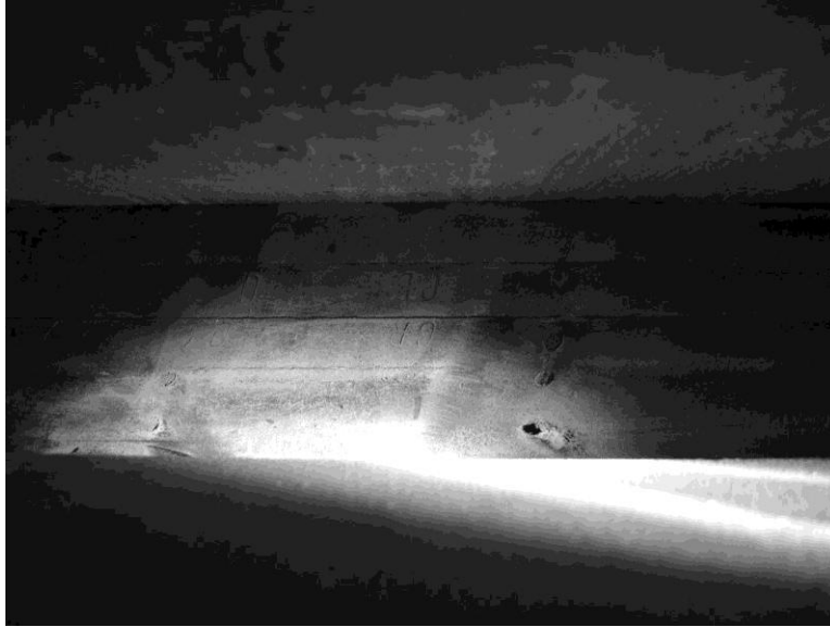
Figure 5.73 – Hairline Surface Cracks on Elastomeric Bearing
