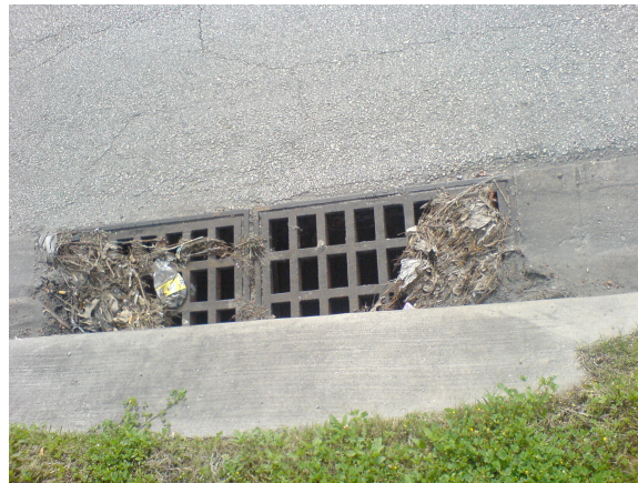
Figure 8: Image of Curb and Grate inlet with debris residue. Image is from a municipal street, but illustrates the debris issue as well as typical grate sizing.
