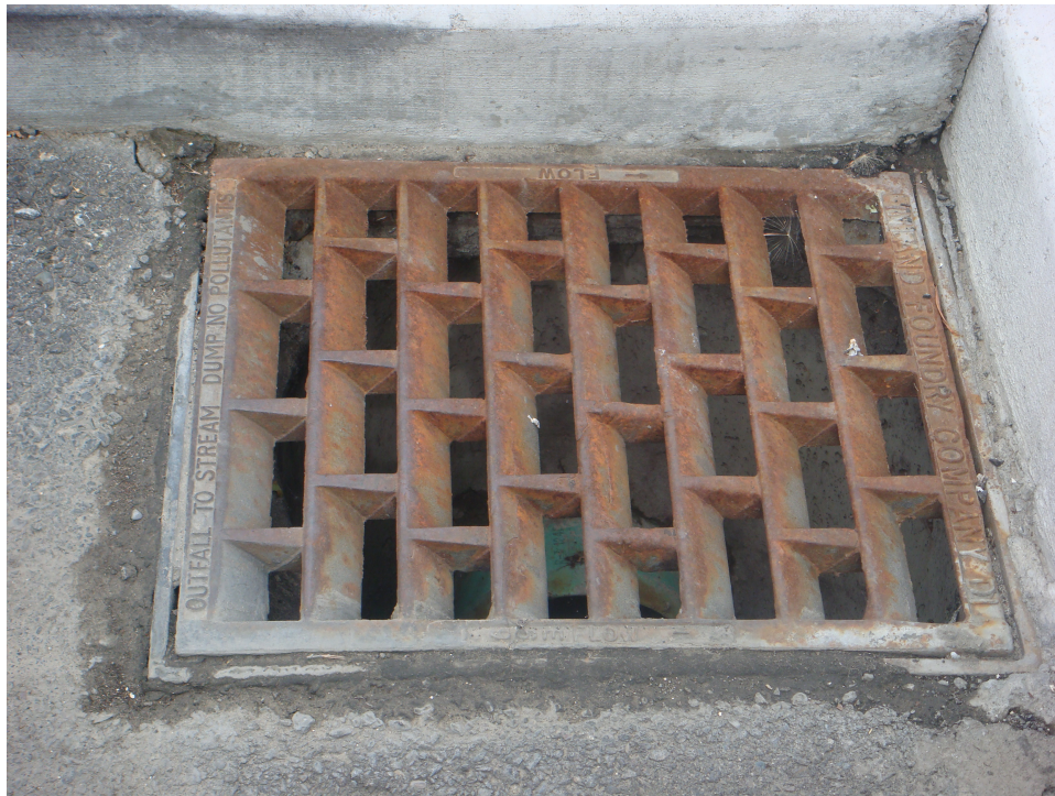
Figure 7: Image of a slanted vane inlet in service.
