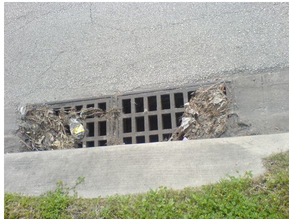
Figure 8: Image of Curb and Grate inlet with debris residue. Image is from a municipal street, but illustrates the debris issue as well as typical grate sizing.
