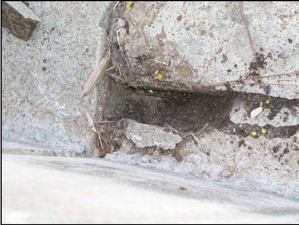
Figure 5.10 An Access Point for Intrusion of Bridge Surface Water Runoff
