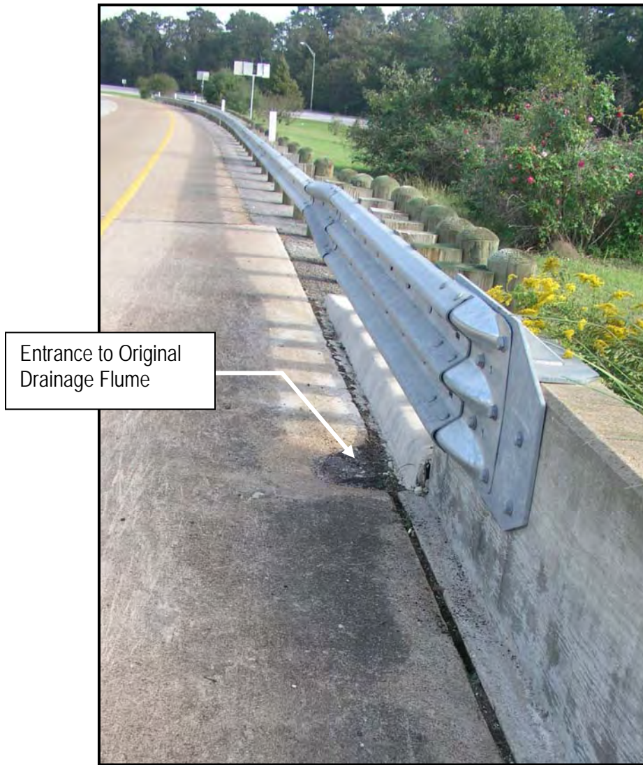
Figure 5.8 Entrance to Original Drainage Flume Blocked by the Installation of the Monocurb in the New Thrie Beam Guardrail System
