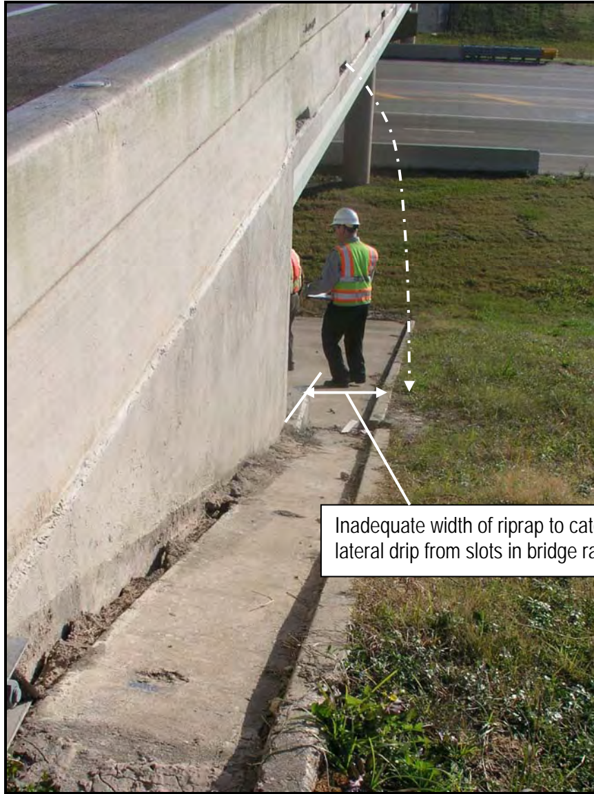
Figure 5.5 Inadequate Riprap Width (Houston District)
