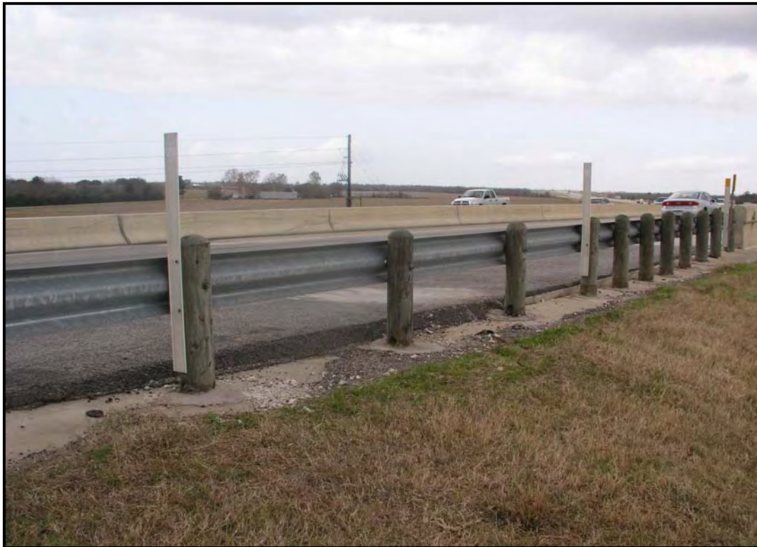
Figure 5.16 Multiple Overlays Used to Remedy Bridge End Settlement
