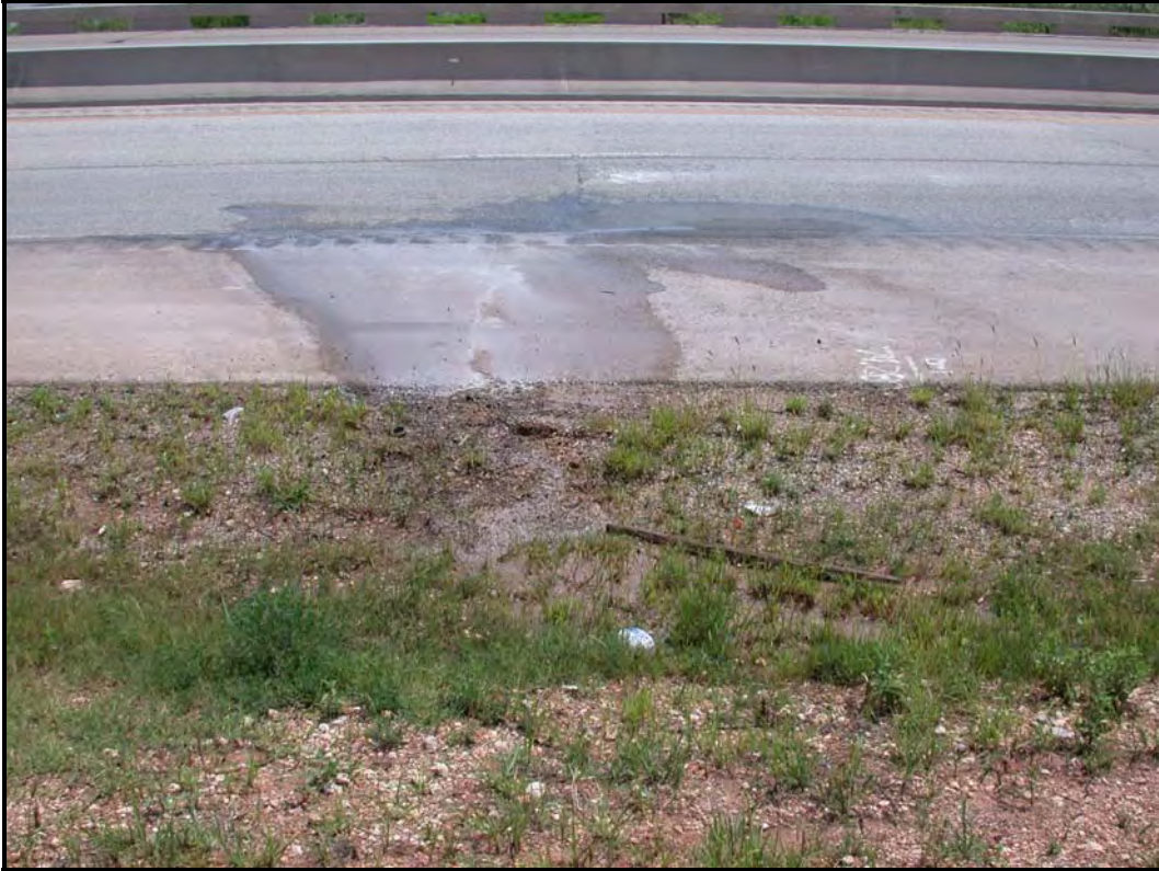
Figure 5.3 Water Seepage at the US-83 Overpass Bridge Departure over Antilley Road in Abilene District
