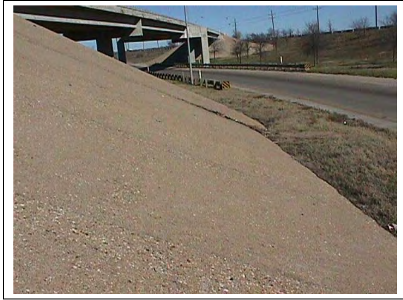
Figure 4.4 Differential Settlement of Riprap Slab (Side View)
