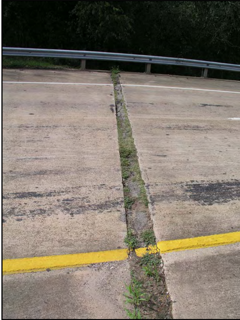
Figure 5.9 Poorly Maintained 5-inch Wide Joint between Bridge Deck and Approach Slab
