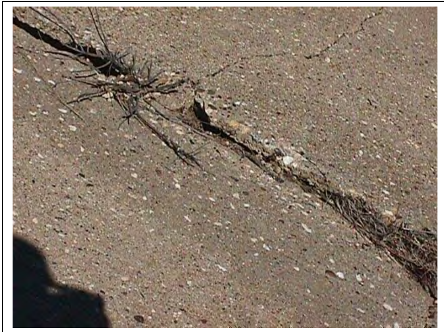
Figure 4.3 Damaged Joint in Riprap Slab
