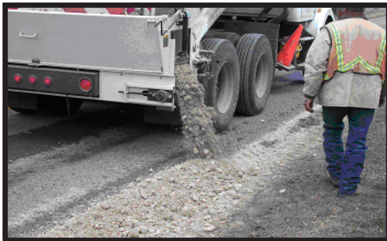
Figure 5. Edge maintenance equipment includes conventional, in-house-modified, and commercially manufactured equipment specifically dealing with pavement edge drop-offs.
