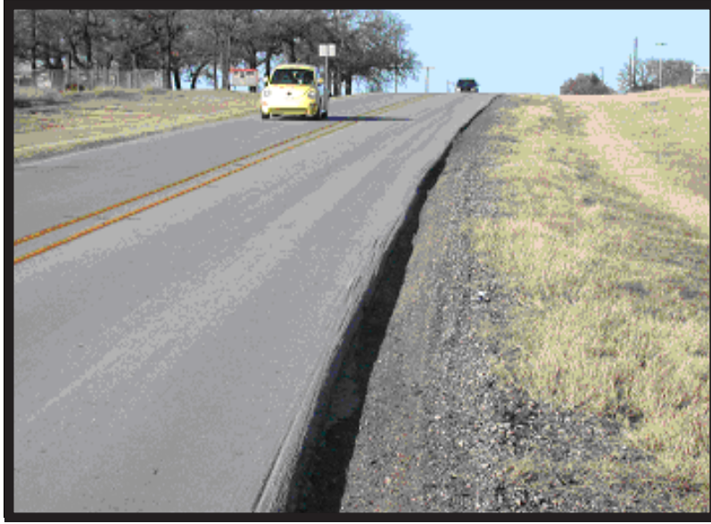
Figure 2. Maintenance personnel define edge drop-offs in risk-based terms with respect to two functional criteria: 1) the impact on safety of the traveling public, and 2) the potential for damage to the road.
